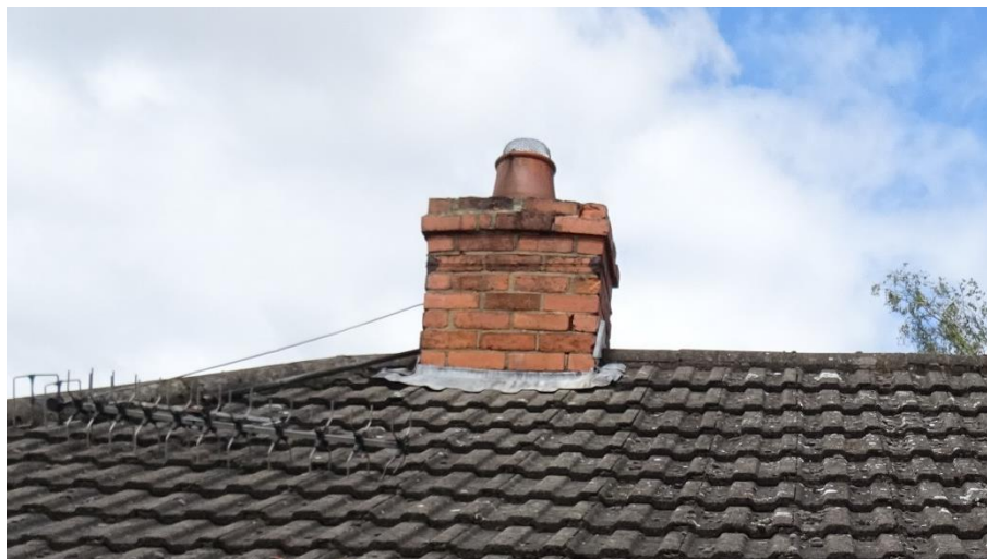
Figure 4.8. Leadwork with some gaps beneath
