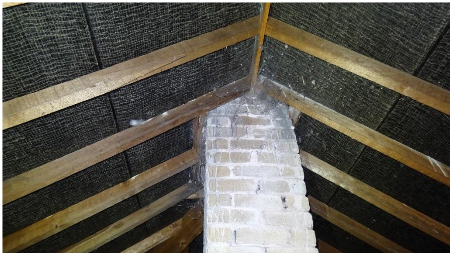
Figure 4.6. Roof lining and cobwebbing
