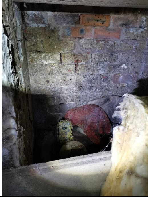
Photograph 19: The static detector in situ in the basement.
