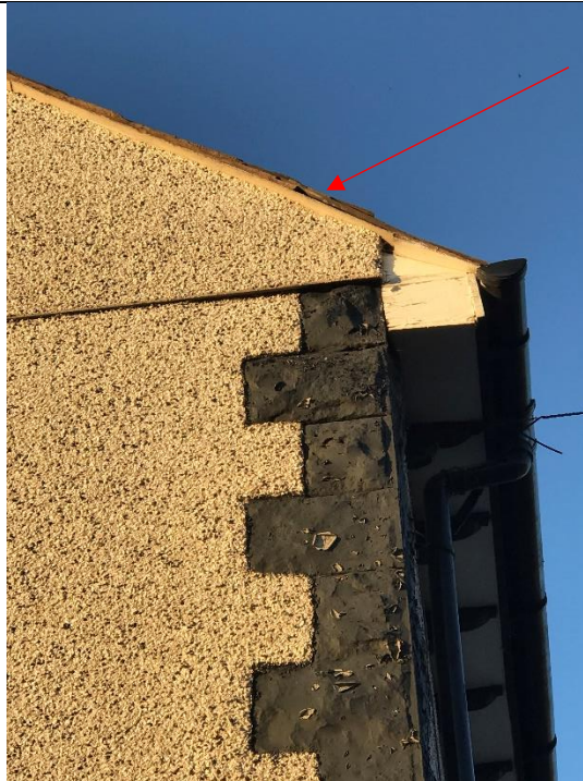
Photograph 10: Missing mortar on the west gable end of the property. (TN2)
