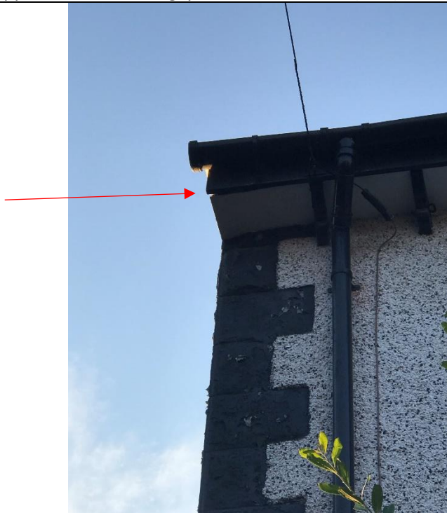
Photograph 4: The front aspect, with association to the west gable wall of the property showing the gap in the soffit box.
