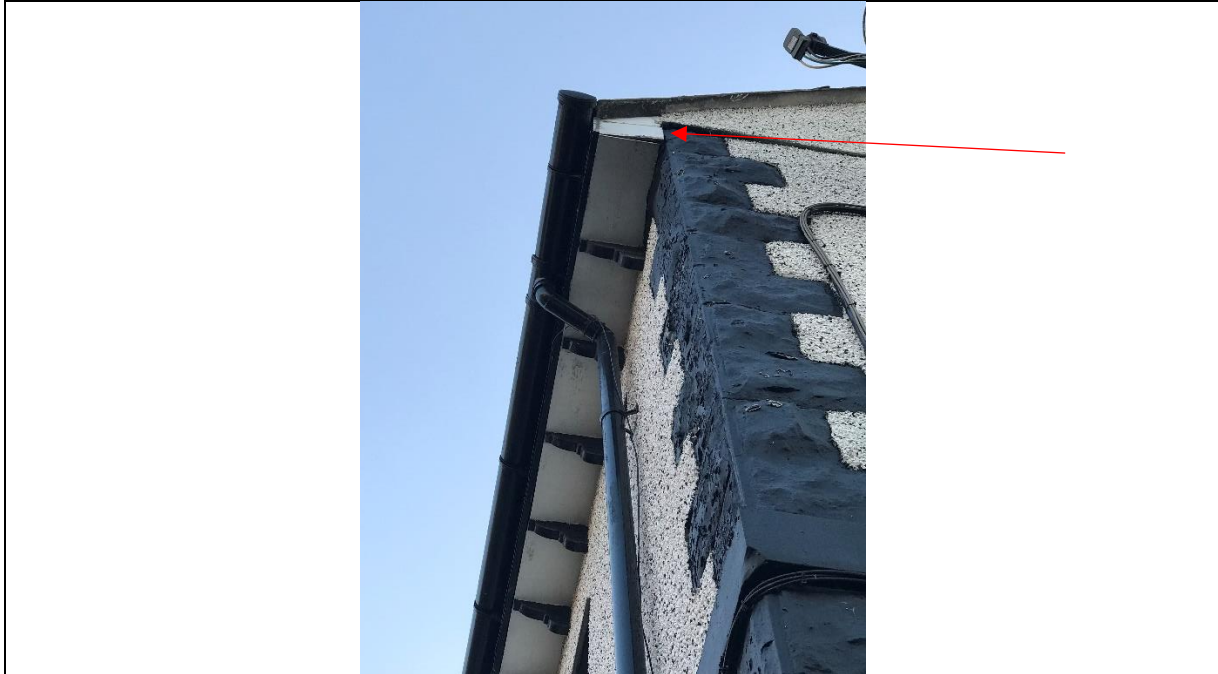
Photograph 5: The front aspect, with association to the east gable wall of the property showing the gap in the soffit box.
