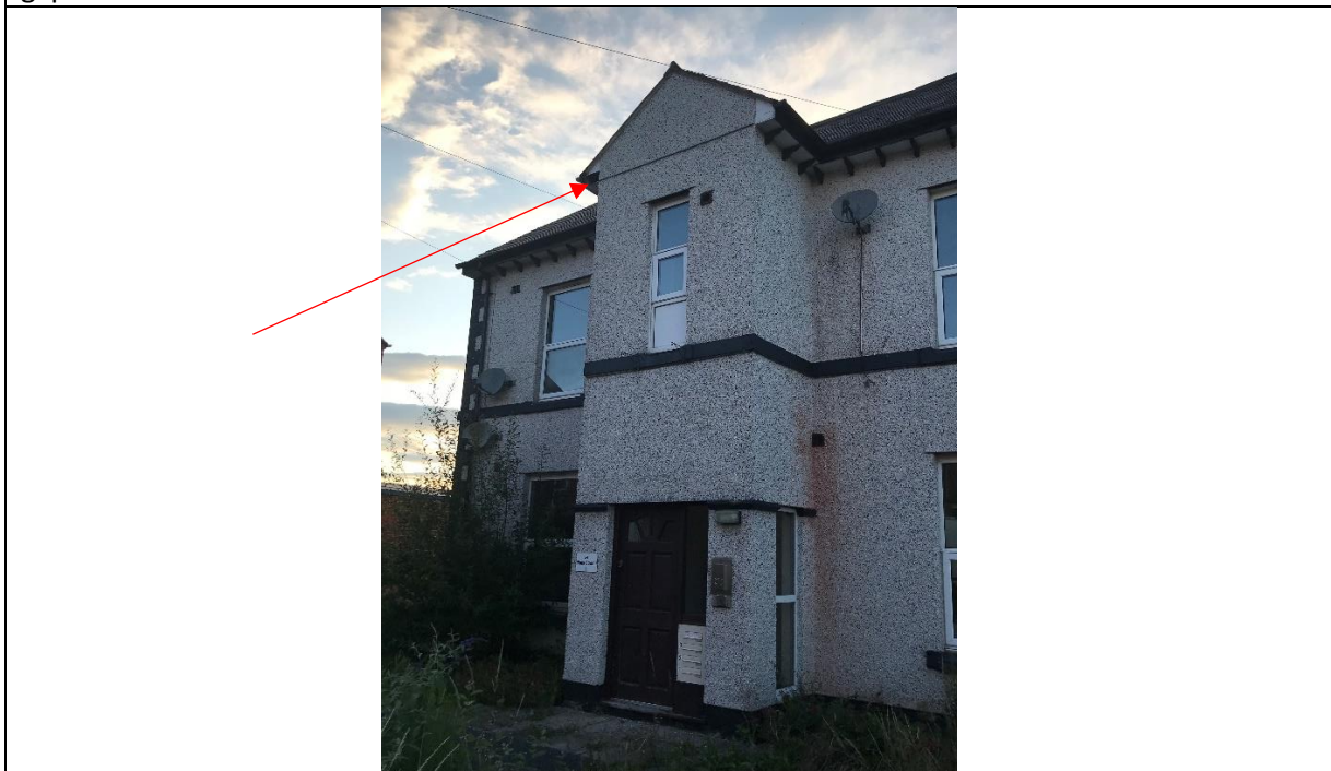
Photograph 6: Missing end of the soffit box, possibly only been missing for a couple of days at the time of writing. (TN3)
