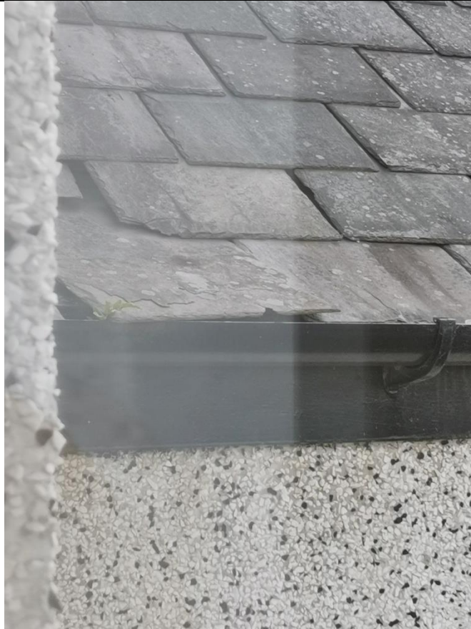
Photograph 3: A slipped slate tile with gaps, on the rear roof (TN1).
