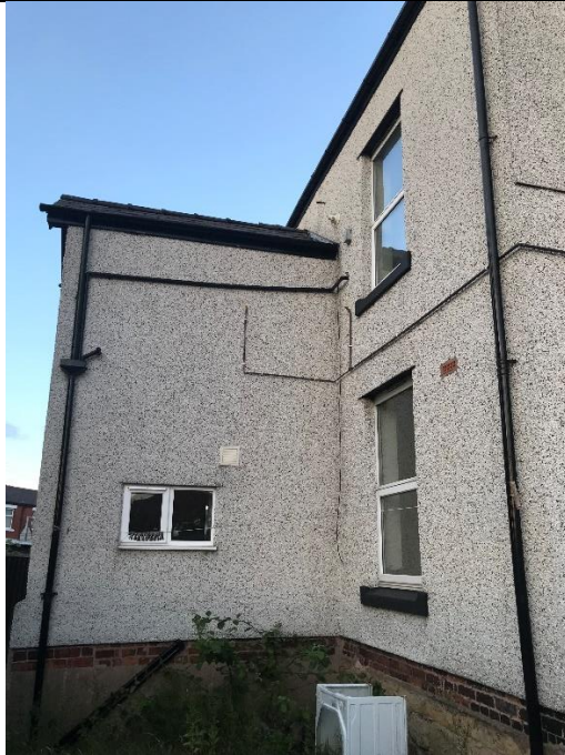
Photograph 9: Facia boards at the rear of the property.
