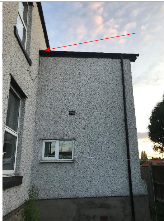
Photograph 8: Facia boards at the rear of the property. Arrow is pointing to where the slipped slate roof tile was. (TN1)
