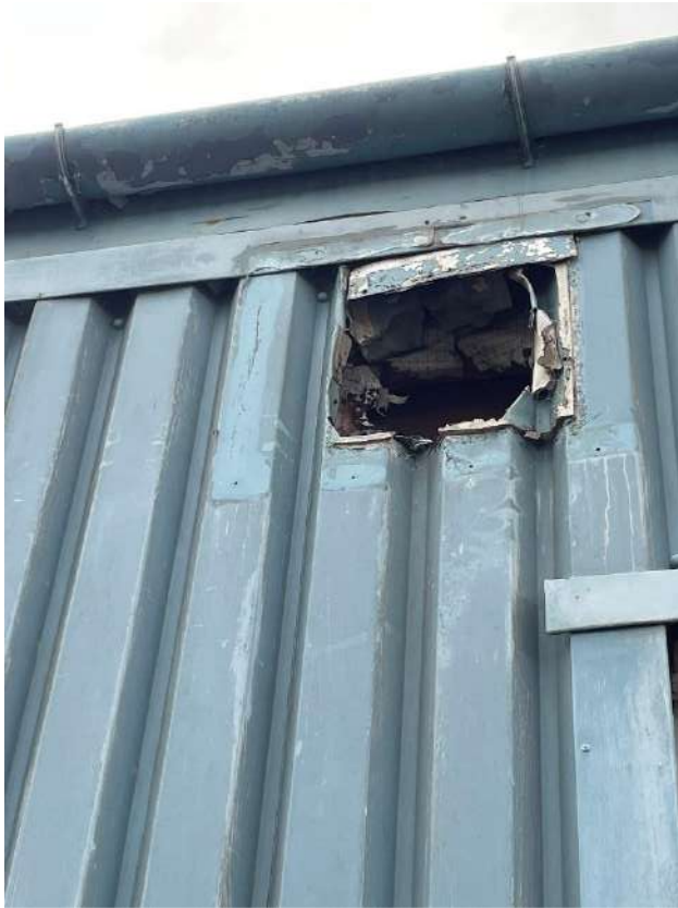
Photograph 15. A hole within the corrugated, galvanised metal on the north-western aspect of Building 4.
