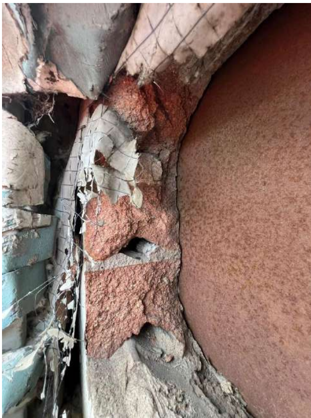
Photograph 16. The south-western facing cavity in the brickwork on Building 4.
