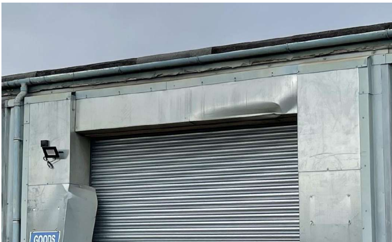
Photograph 12. The gaps underneath the fascia board on the south-eastern aspect of Building 4.
