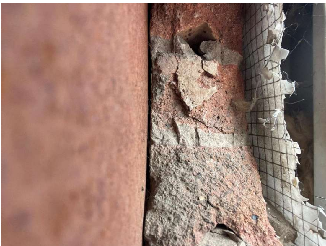
Photograph 17. The north-eastern facing cavity in the brick work on Building 4.
