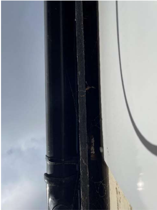
Photograph 19. The gap underneath the wooden barge boards on the extension of Building 4.
