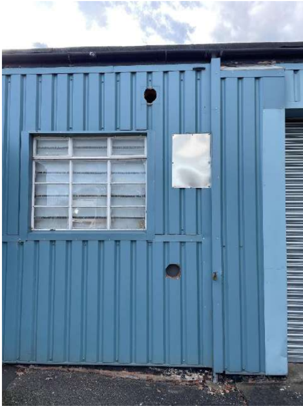
Photograph 7. A hole in the corrugated, galvanised metal on the north-eastern aspect of Building 3.
