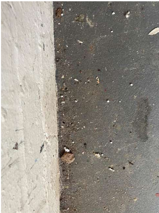
Photograph 26. Mouse droppings inside of Building 4.
