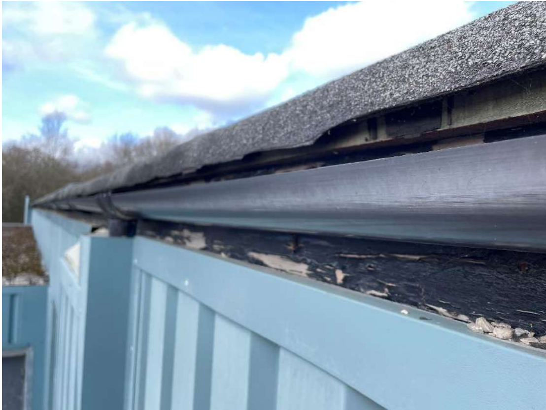
Photograph 5. Raised bitumen felt on the south-western aspect of Building 3.
