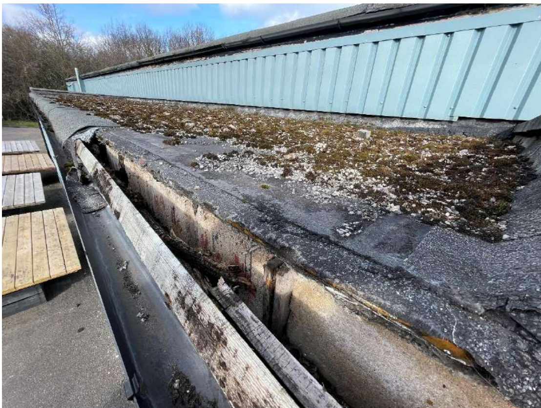
Photograph 6. The rotten wood and lifted bitumen on the south-western aspect of Building 3.
