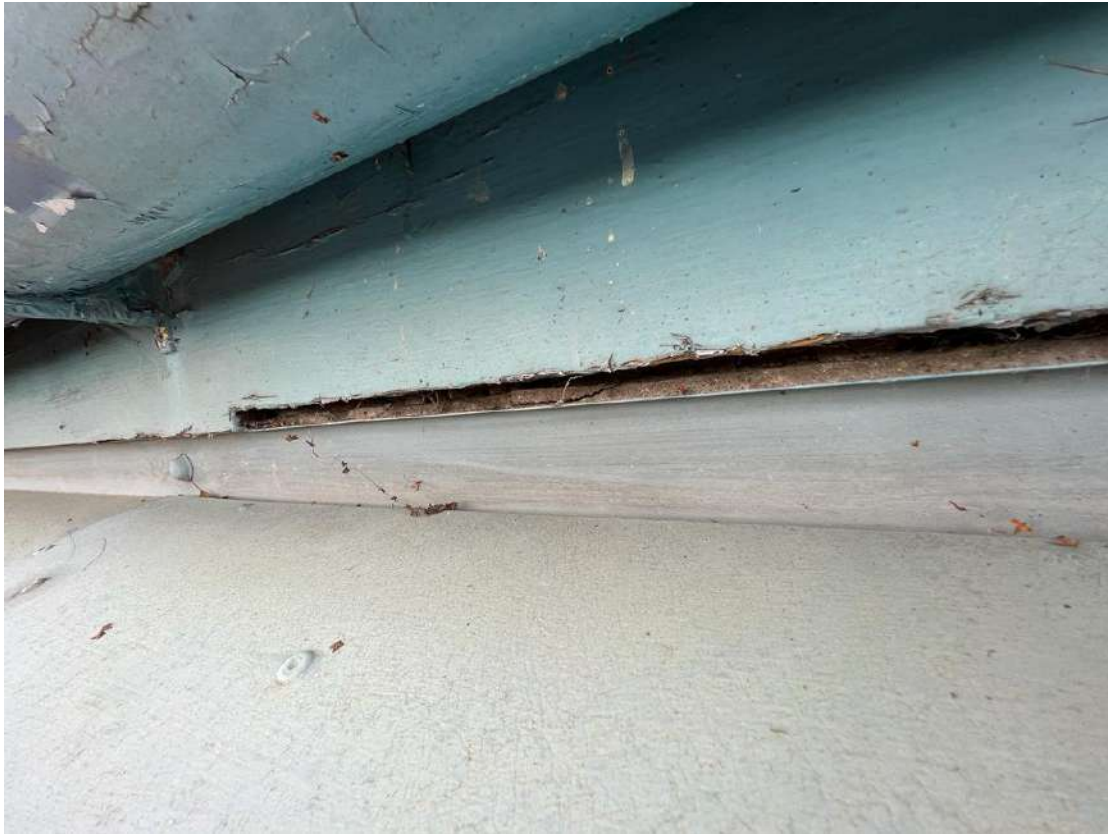
Photograph 13. The sealed gap in the fascia board on the south-eastern aspect of Building 4.
