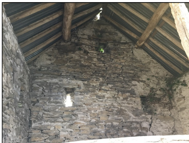
Plate 3 Internal wall crevices are numerous
