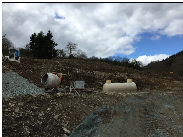
Plate 5 All semi-natural habitats within site have been cleared
