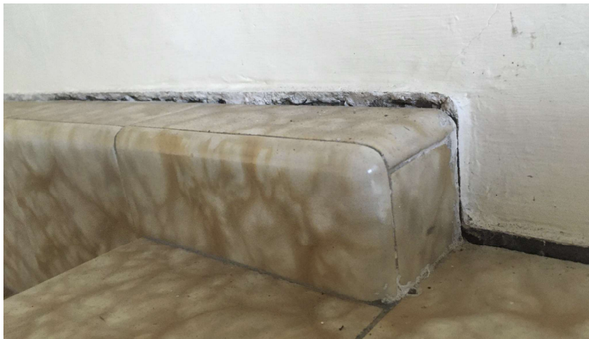
Figure 4 - Detail showing movement of fireplace due to overloading of floor
