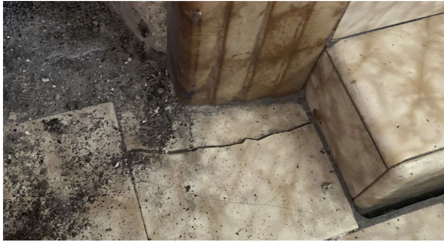
Figure 5 - Detail showing movement of fireplace due to overloading of floor
