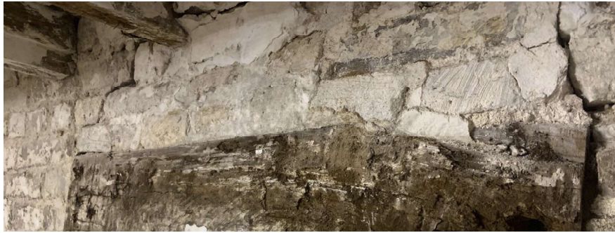
Figure 3 - Structural failure below fireplace
