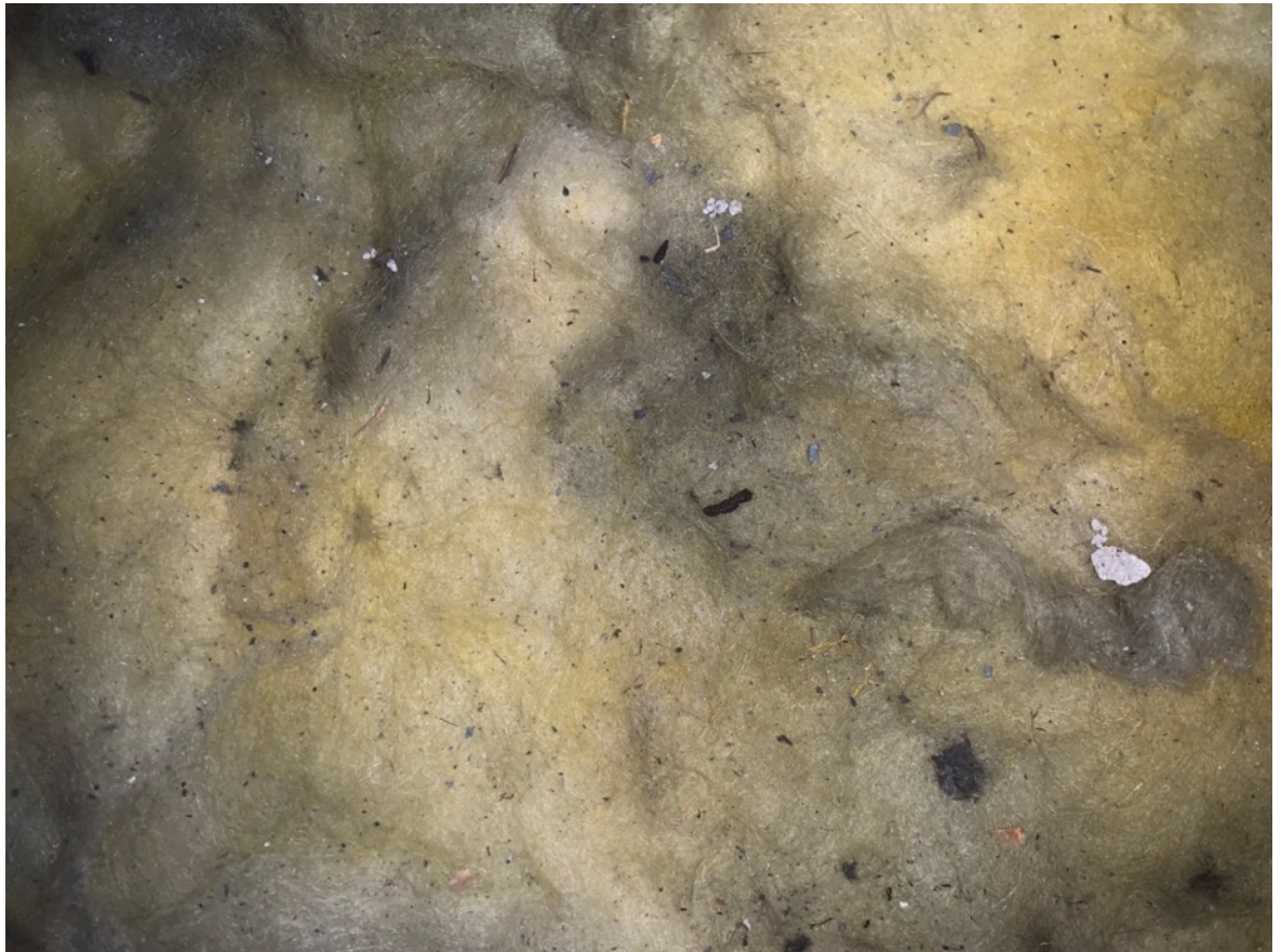
Photograph 4. Bat dropping within roof void
