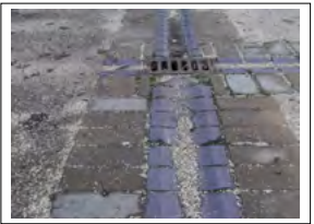
Photo WCM05 - museum courtyard gulley
