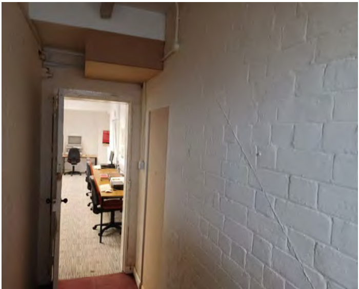
Several historic doorways such as this will be too narrow for use as an accessible entrance
