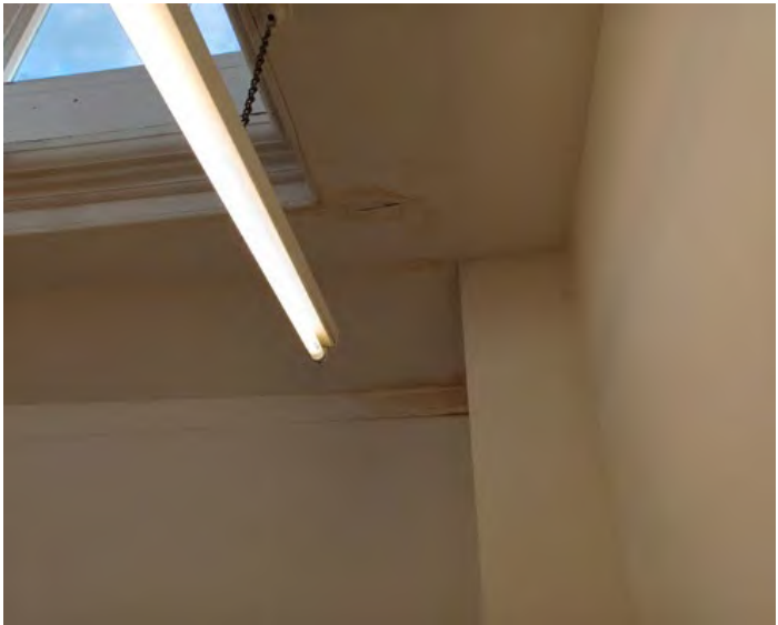
Leaking gutters causing water ingress
