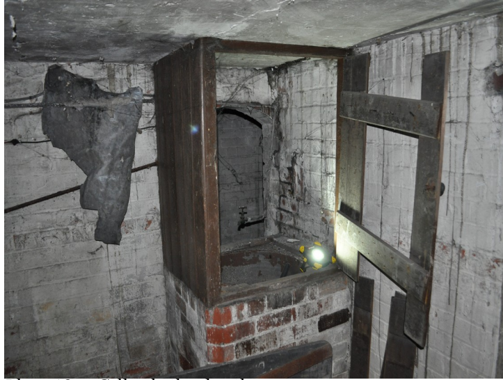
Plate 43 - Cellar boiler detail
