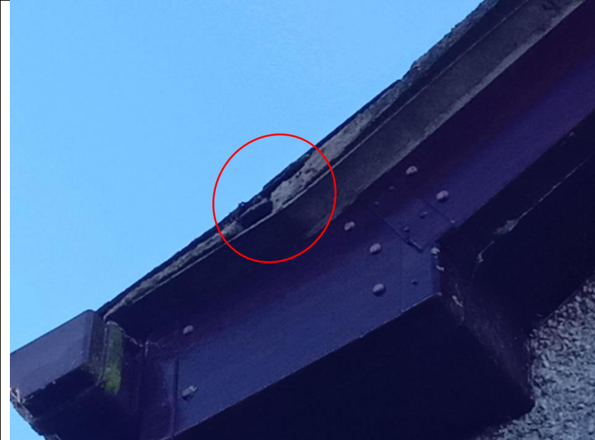
B1 – eastern elevation – missing mortar
