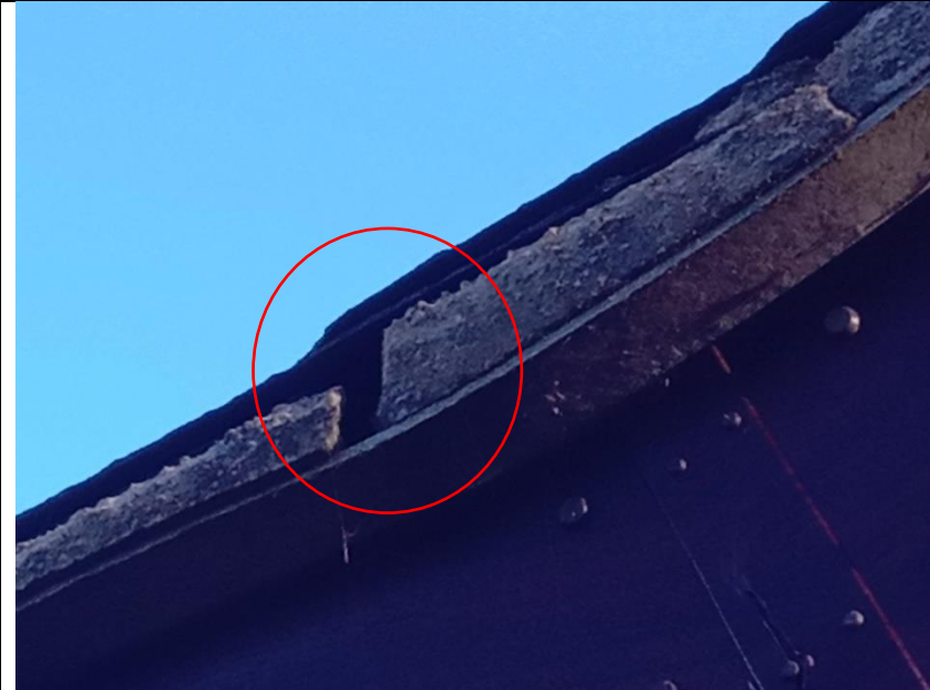
B1 – western elevation – missing mortar
