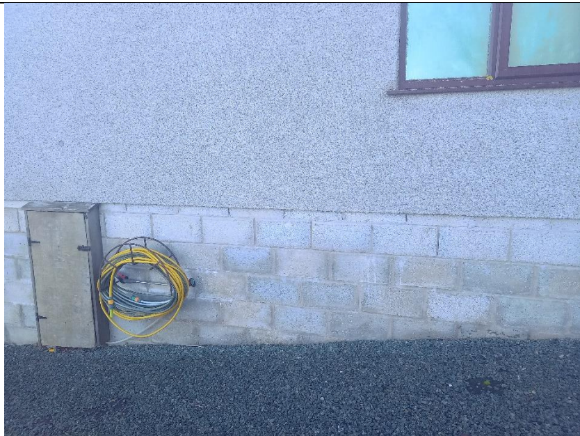
B1 – northern elevation – breezeblocks and pebbledash intact
