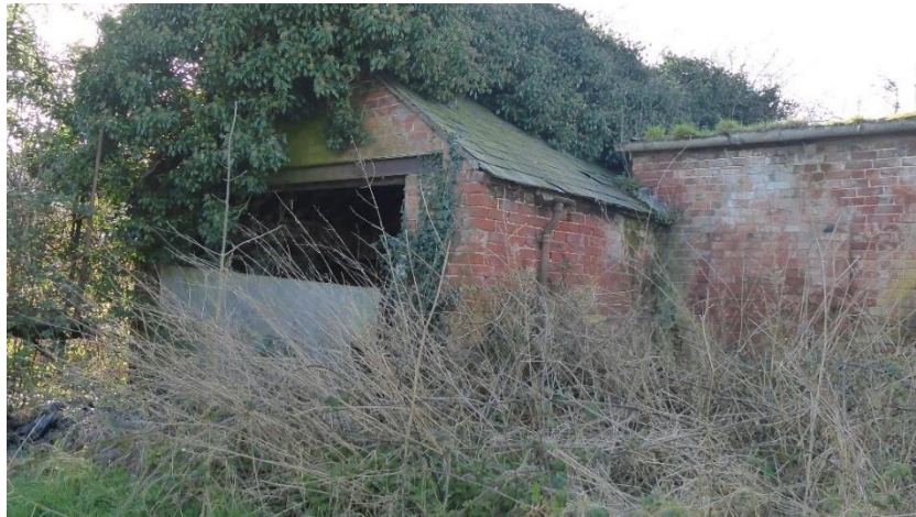
Figure 4.23. Gaps between tiles
