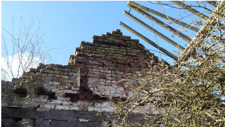
Figure 4.20. Crack and crevices in walls
