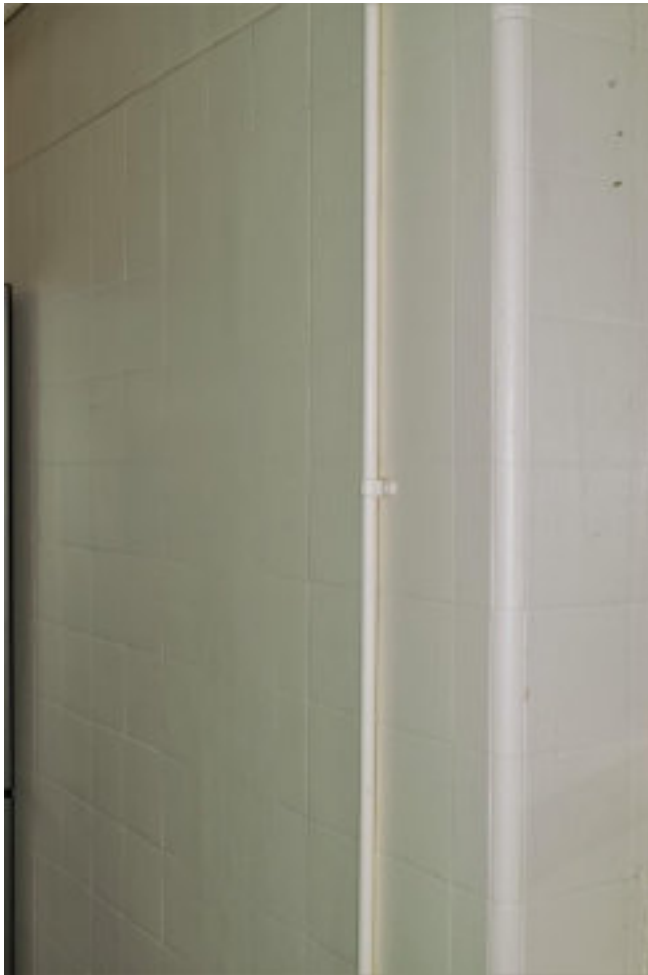
Figure 188 SU R1 Over-painted tiles on wall.
