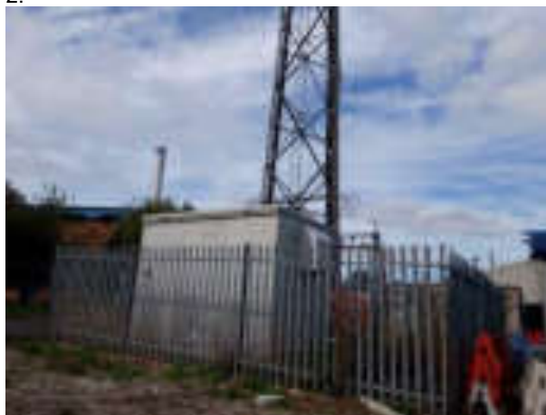
13.09.22 – Electricity pylon with small metal structure.
