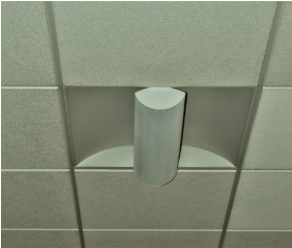
Figure 88 Restaurant SE section light fitting detail.
