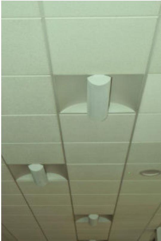
Figure 86 Restaurant SE section light fittings.
