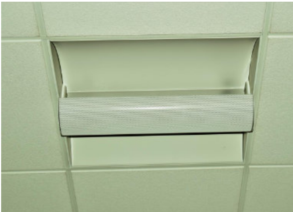
Figure 89 Restaurant SE section light fitting detail.
