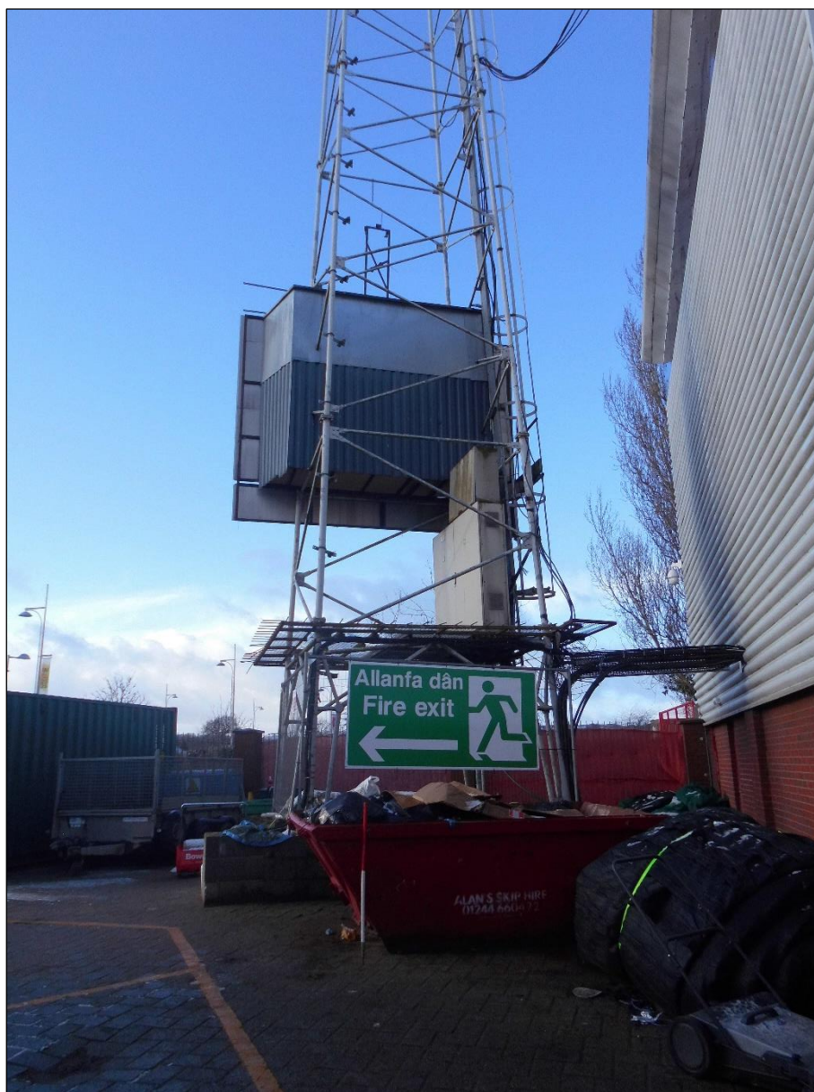
Plate 20: Close up of generator on Floodlight B (same as others), looking W. 1m scale.
