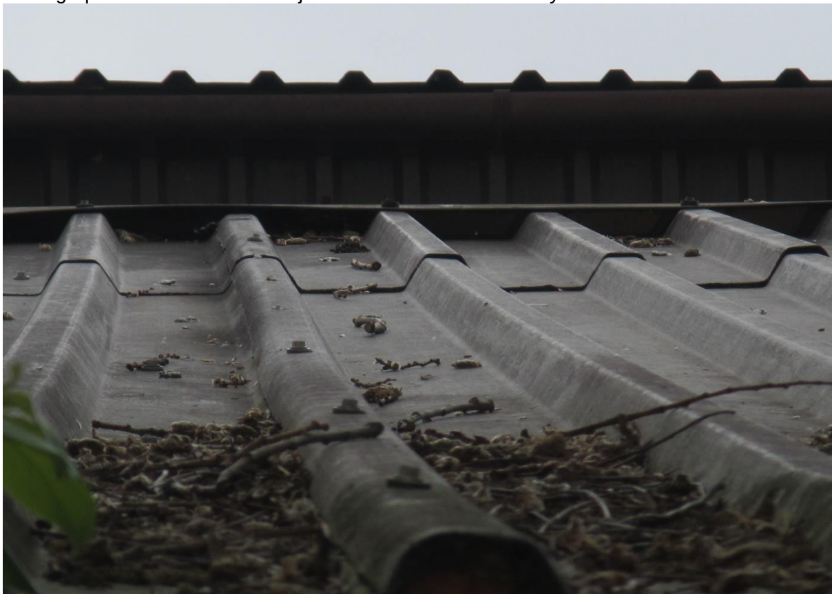
Photograph 12 – Gaps beneath the ridgeline.
