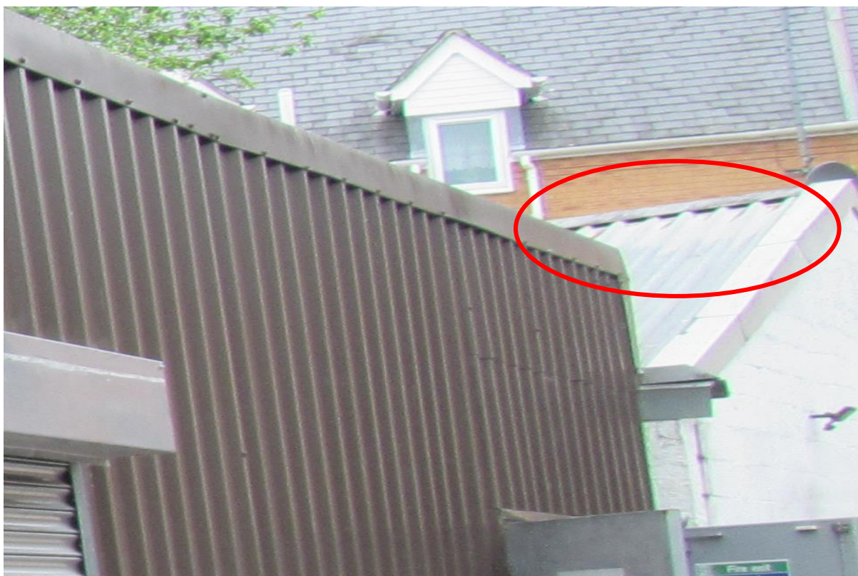
Photograph 2 – Gaps below the ridge line.
