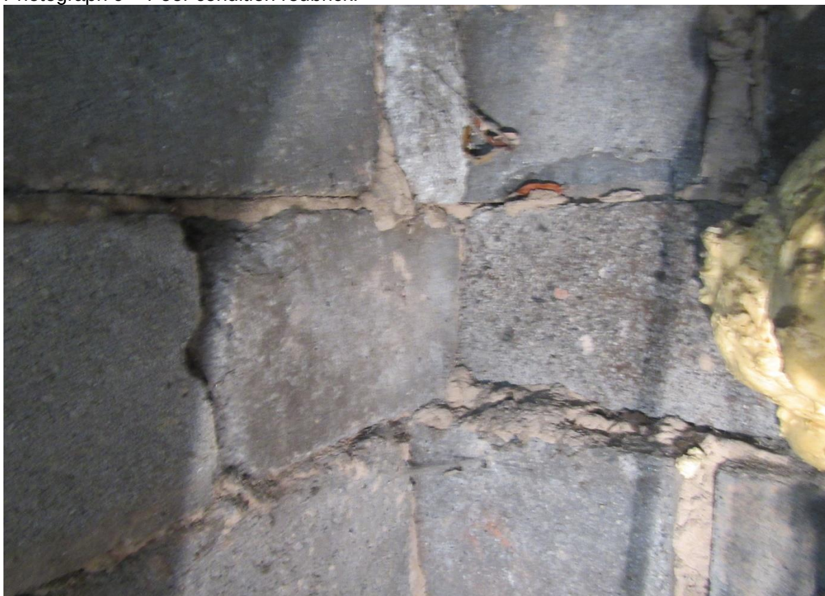
Photograph 10 – Gaps in the breezeblock mortar.
