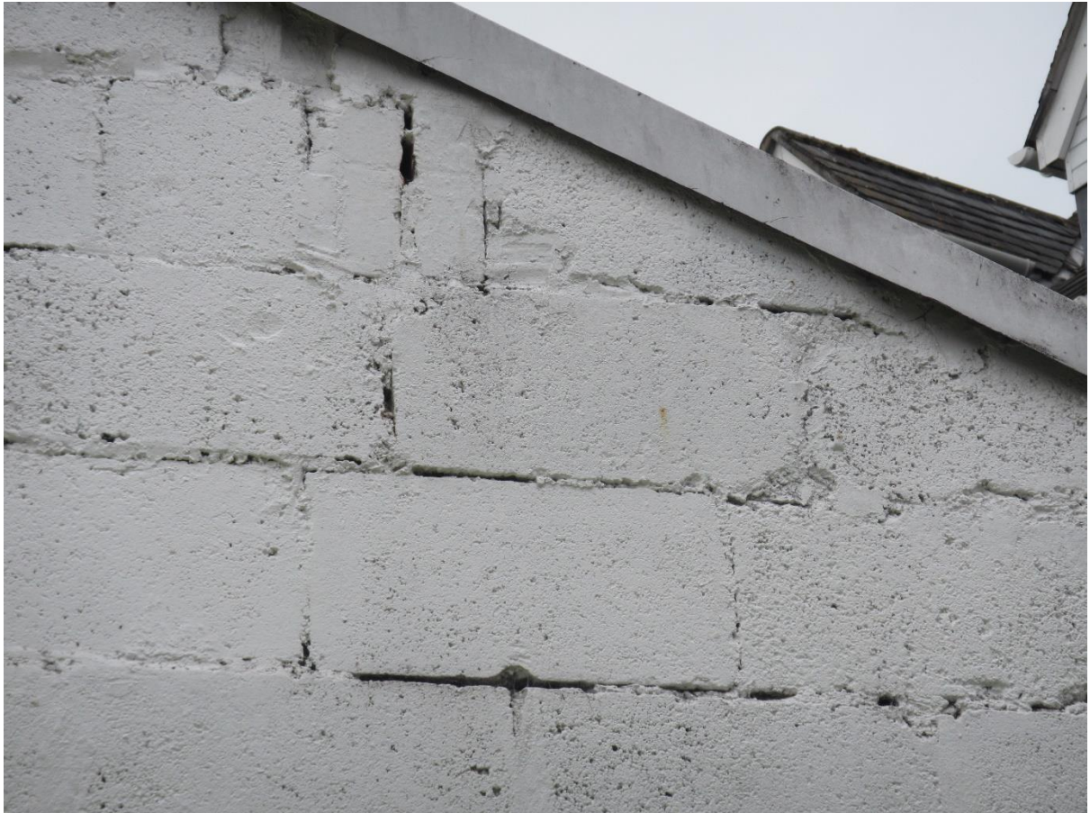
Photograph 5 – Gaps between the breezeblocks of the bakery.
