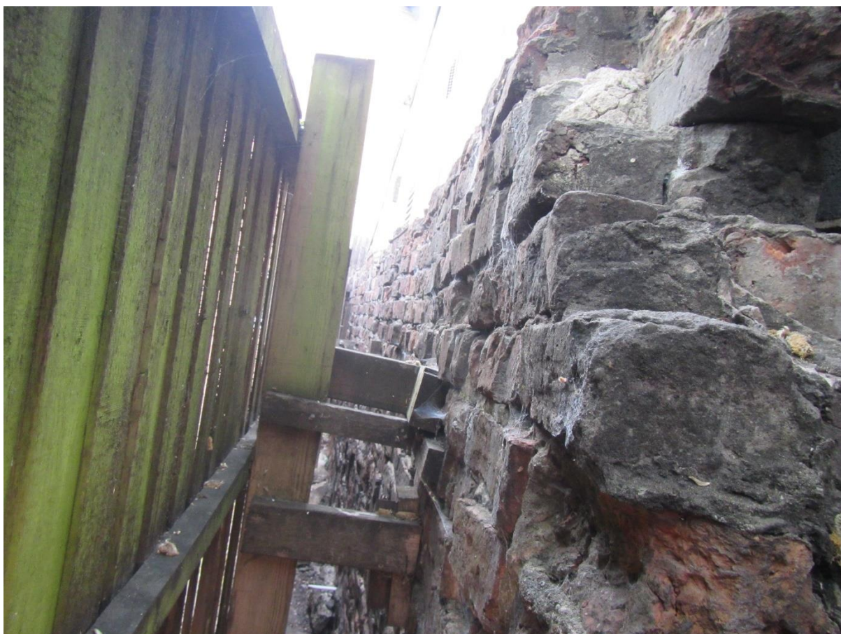
Photograph 9 – Poor condition redbrick.
