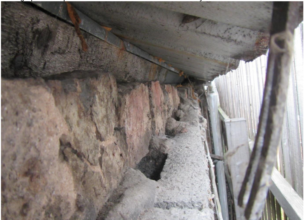
Photograph 6 – Crevices between the breezeblock and redbrick on the north-eastern aspect.
