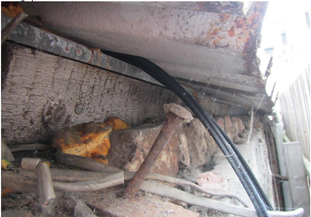
Photograph 4 – Gaps at the eaves on the north-eastern aspect.
