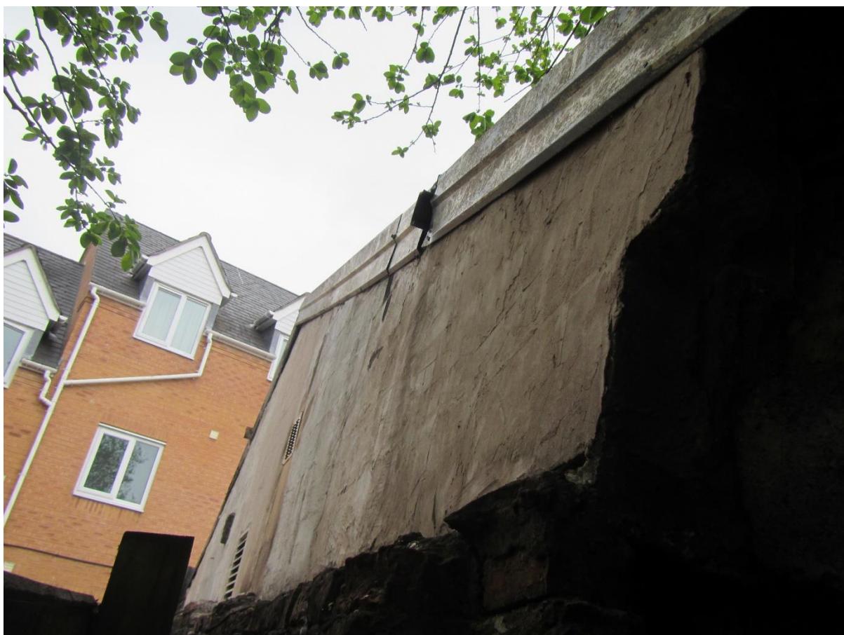
Photograph 7 – Lifted timber fascia.
