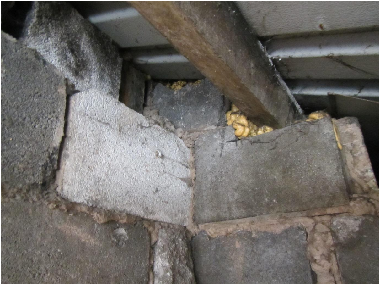
Photograph 11 – Crevices at the junctions between the bakery and warehouse.
