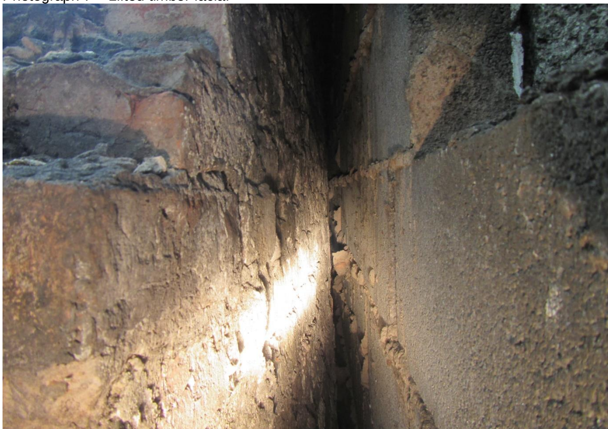
Photograph 8 – Gap between unrendered breezeblock and redbrick.
