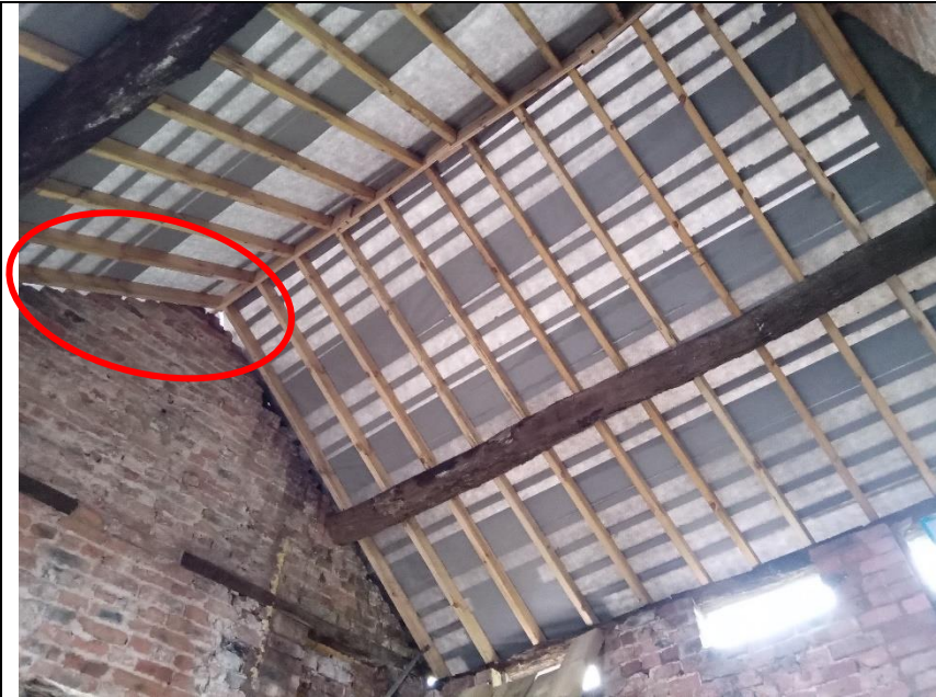
B1 – (interior loft space 1) (gaps in brickwork)
