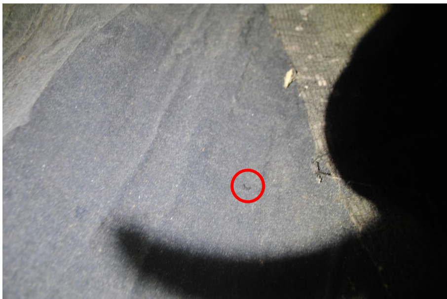
Figure 3.21. Bat dropping seen on new material in new loft area Feb 2023
