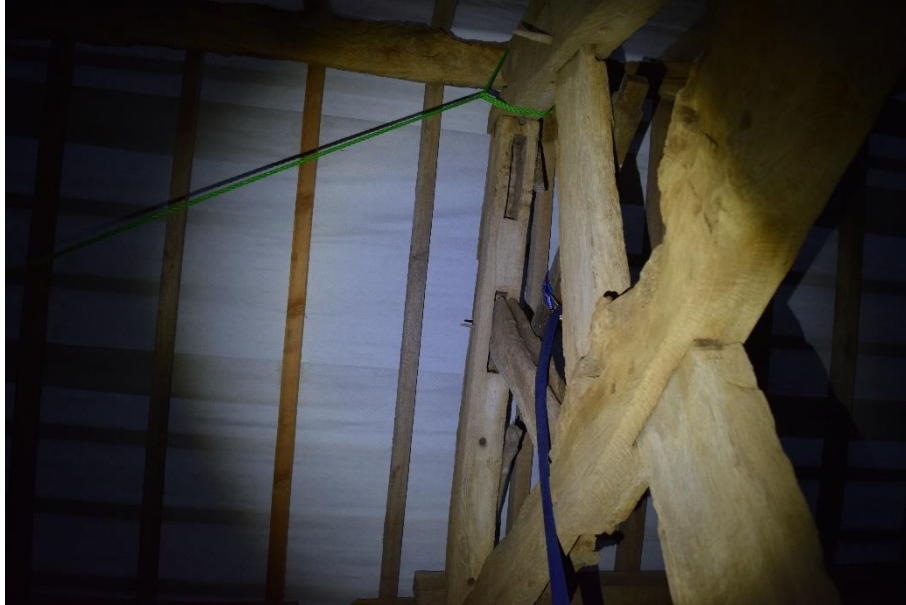
Figure 3.6. Open mortice joint in roof timbers (Feb 2023)
