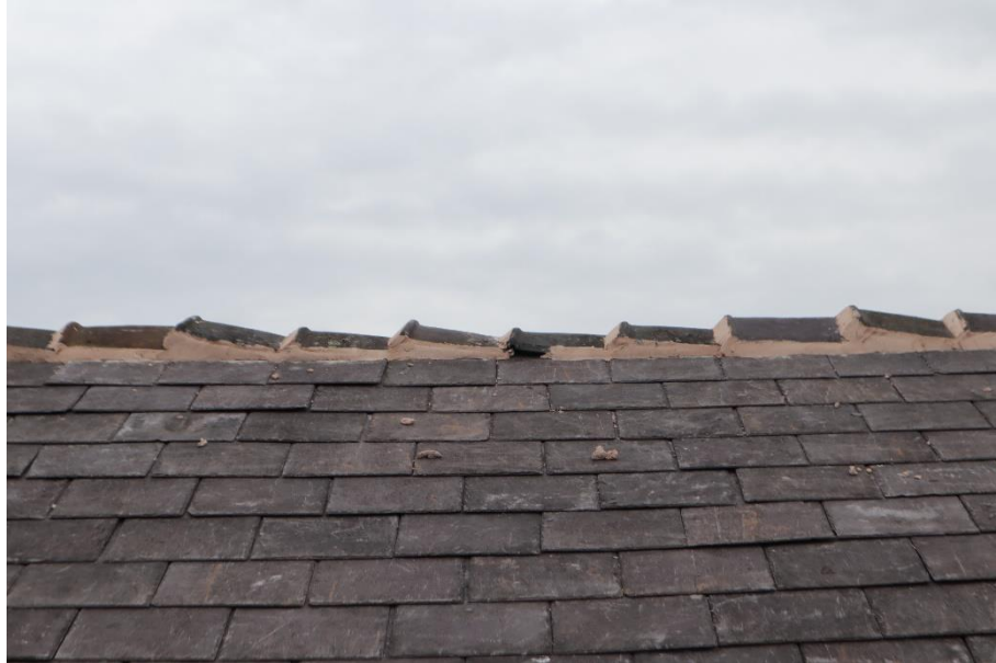
Figure 4.4. Lifted ridge tile
