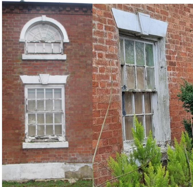
Image 08: Derelict existing windows on front elevation.
