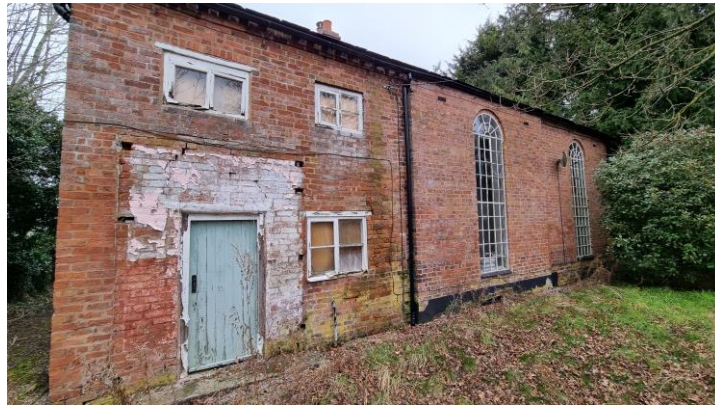
Image 13: Visual evidence of the former extension removed from the rear wall in the position of the proposed extension.
