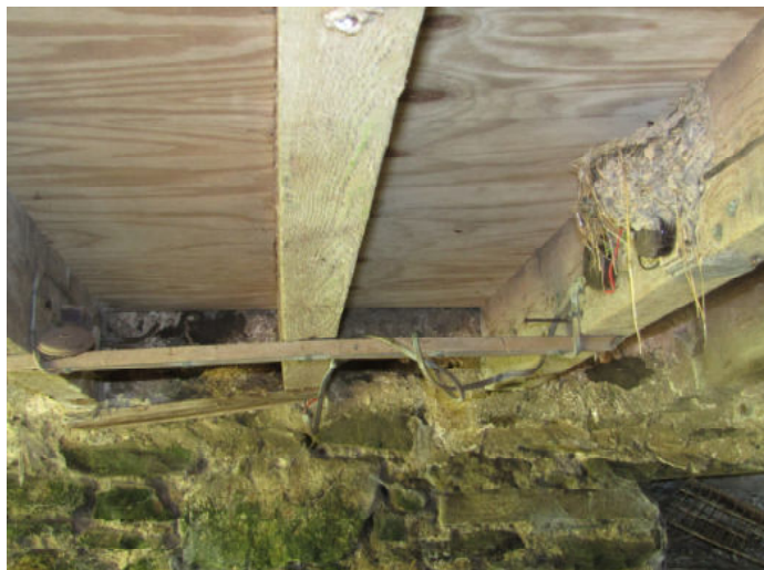
Photo 4: Swallow nest on timbers in ground floor area.
