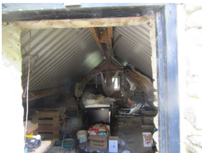
Photo 5: No felt or insulation beneath roof sheets in upper room.
