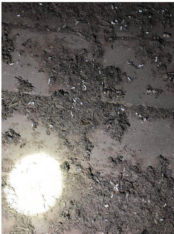
Plate 5 – Abundant bird droppings within the loft
