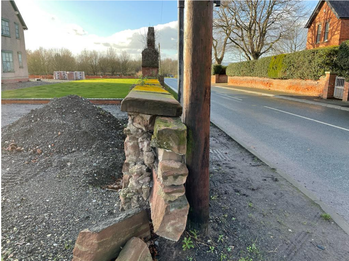
Current Condition of Wall – Leaning substantially towards Roadway
