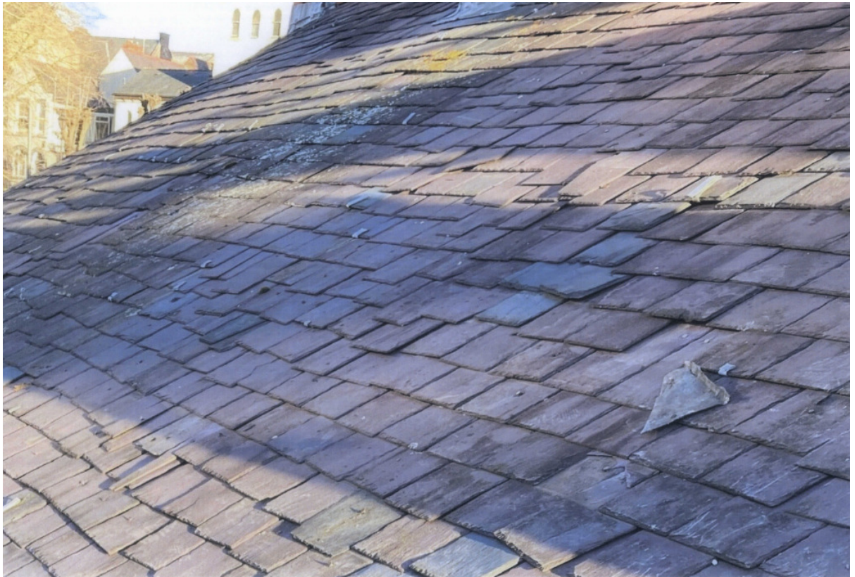
Wider image of the former condition of the roof slates showing slipped and missing slates and slipped lead flashing.
