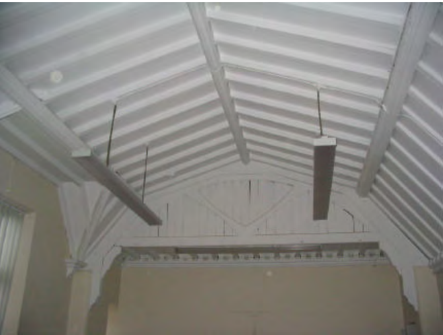
Plate 25 Roof of Court 2, which remains largely as constructed in 1896. Panelling to the far wall (rear of the bench) has been lost.
