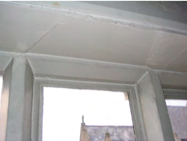
Plate 28 Evidence of former position of partition to F18.
