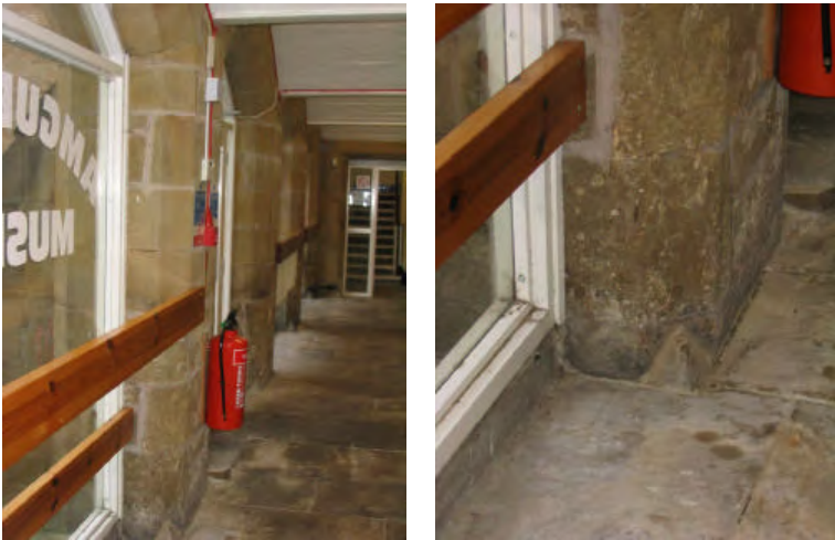
Plate 12 & Plate 13 General view of Loggia, modern screens are clearly visible. On the right the plinth detail has been largely lost as the level of the flags has been raised. The junction of the flags against the plinth suggests that the floor level has been raised, which has created level access into the adjacent office areas. The flags appear to be the originals re-used. The contract provides evidence for this also as it discusses 'stairs into the arcade' and the 'steps out of the doorways into the arcade' (including the sergeant major's quarters) suggesting the original level was probably significantly different. 27
