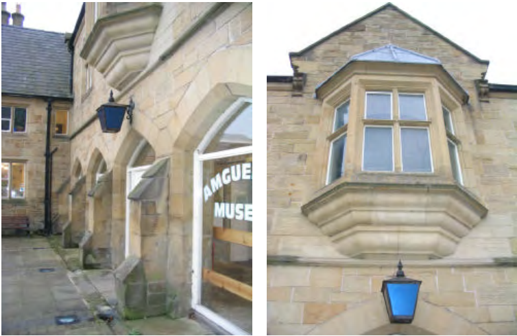
Plate 29 & Plate 30 Loggia, with poor quality modern joinery and Oriel Window.
