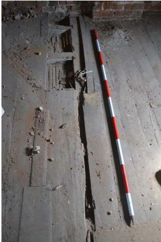
Plate 52: First Floor, Bedroom 2. Damage to deal floor caused by failure of bearer beam below. Scale = 2m.
