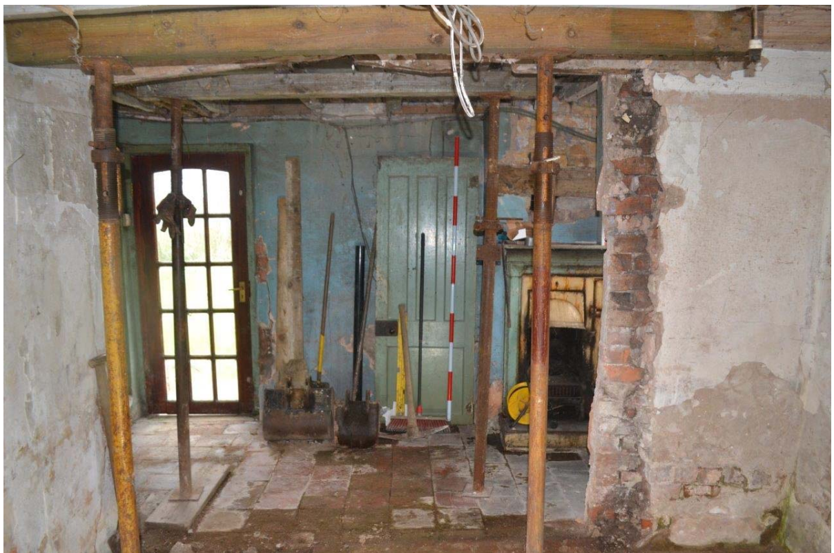
Plate 23: Ground Floor, Private Room. Collapsed wall which once separated the Private Room from the Kitchen. The floor to first floor bedroom above is propped. Scale = 2m
