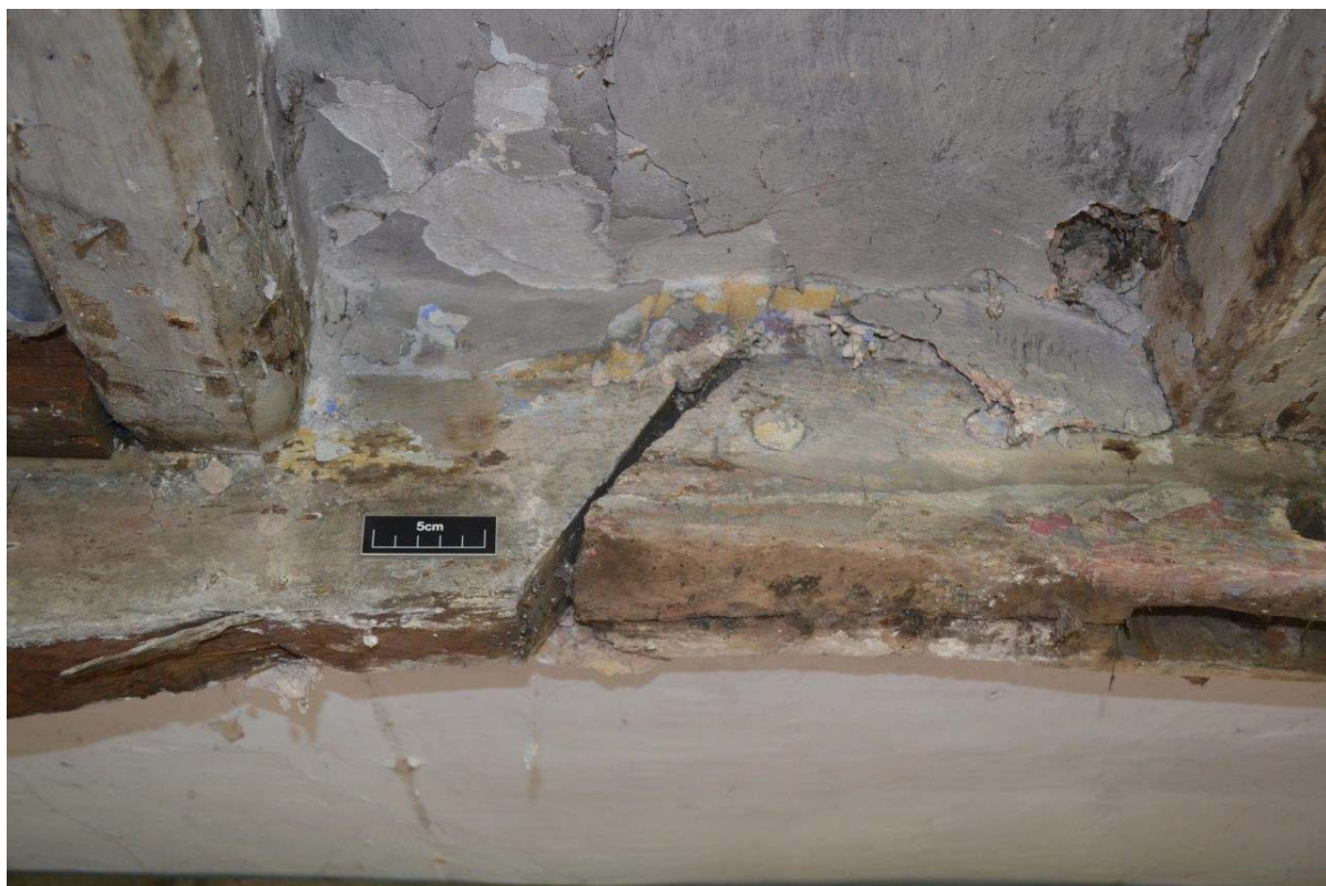
Plate 35: Ground Floor Kitchen. Failure in bearer beam above the (removed) wall separating the kitchen from the private room. Scale = 5cm.
