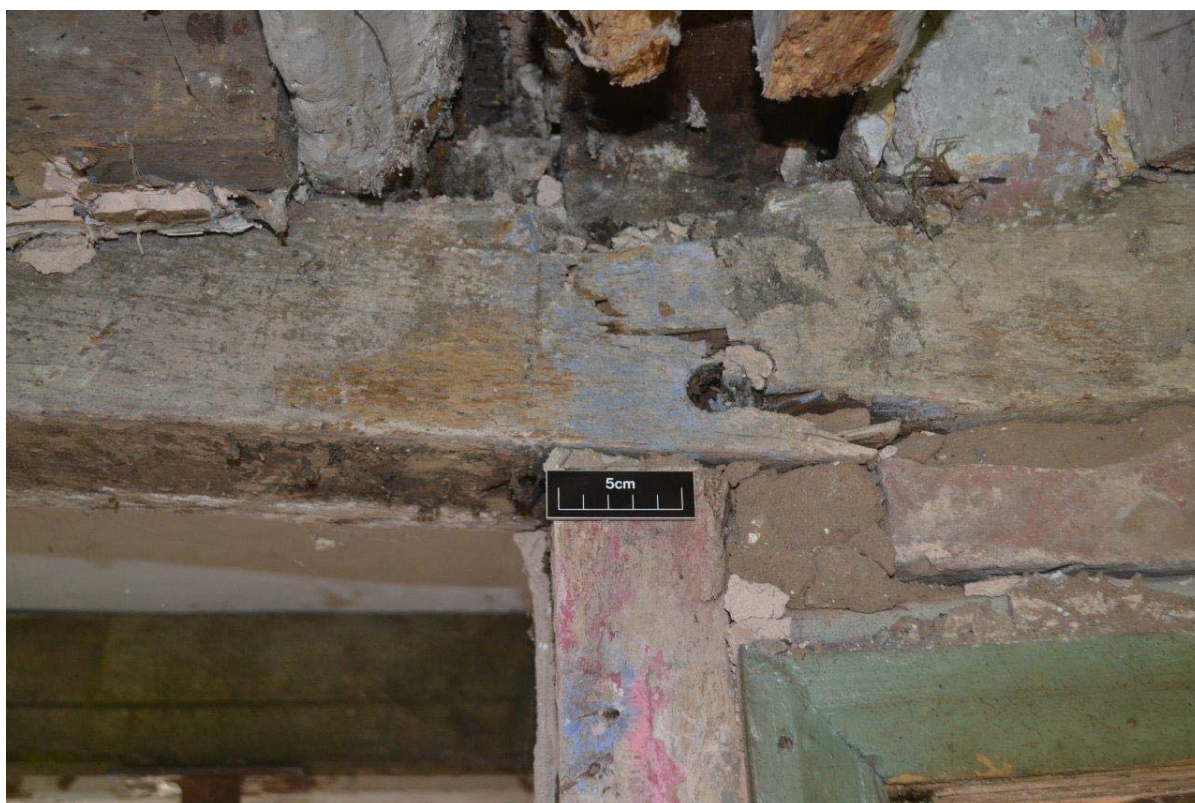
Plate 34: Ground Floor Kitchen. Failure in bearer beam above the (removed) wall separating the kitchen from the private room. Scale = 5cm.
