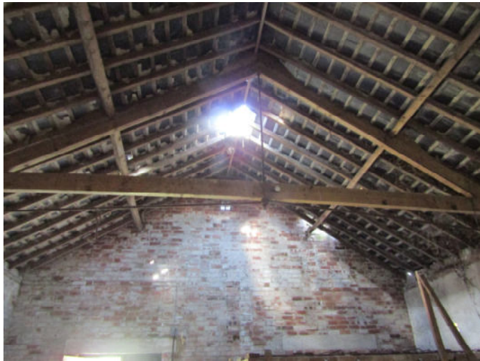
Photo 1: Moderately high level of light penetrating barn via windows and holes in roof.
