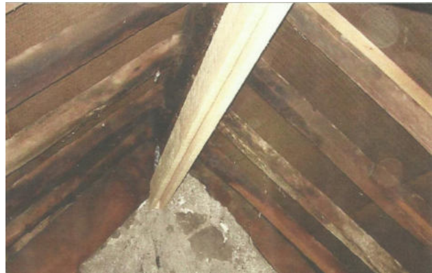
Figure 16: Example of crevice box in a loft void.
