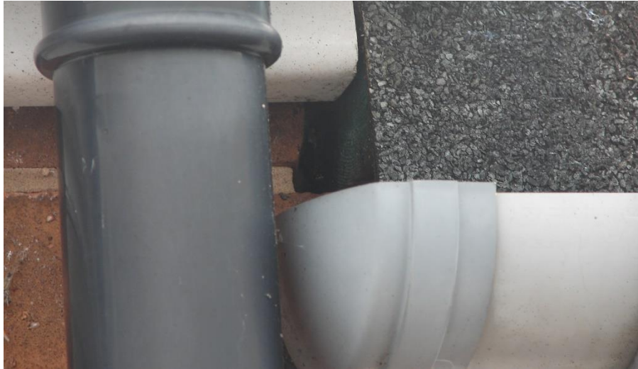
Typical gap between wall (of unit 10) and roof (of unit 11), Target Note 5 .
