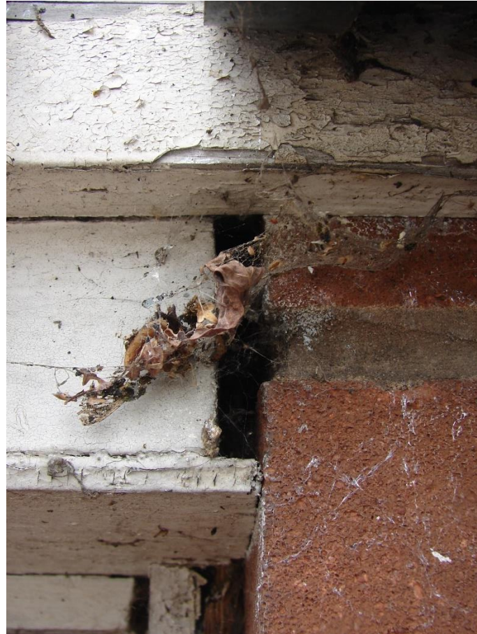
Gap between timber and wall, Target Note 6. Covered in cobwebs.
