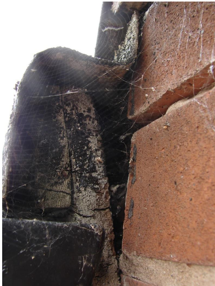
Gap between roof timber and wall, Target Note 6 . Covered in cobwebs.
