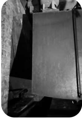
Old oil tank, fire hazard cannot be removed until access points installed
