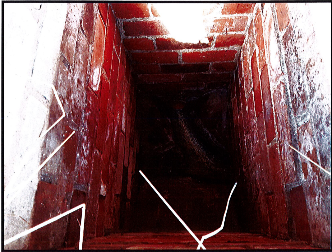
Photograph 3. Manhole chamber for shaft drainage.
