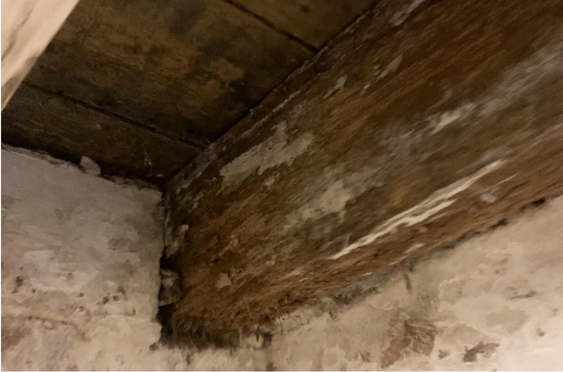
Figure 2 - Existing condition of deteriorated timber joists sitting directly onto brick
