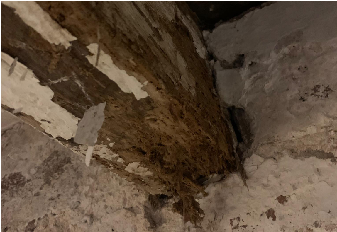
Figure 3 - Additional image of existing joist condition
