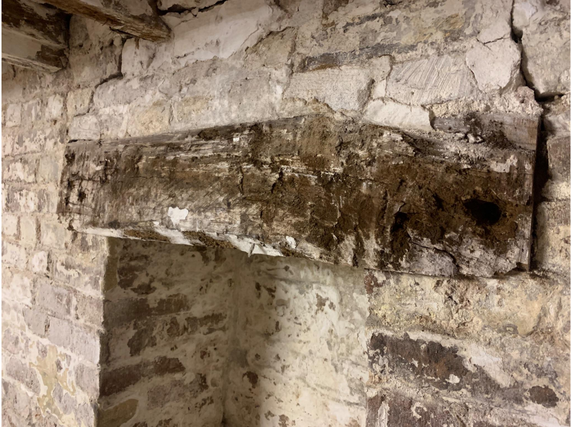
Figure 1 - Existing deteriorated condition of timber lintel
