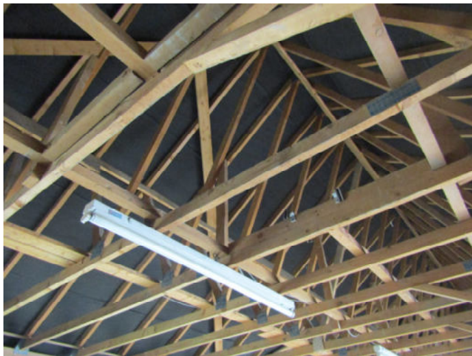
Photo 2: No loft void – roof open to ridge.
