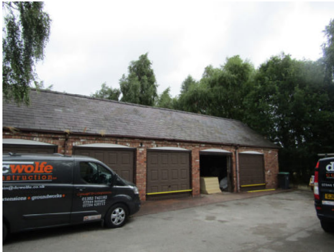
Photo 1: No roofing felt present, timbers smothered in old cobwebs.
