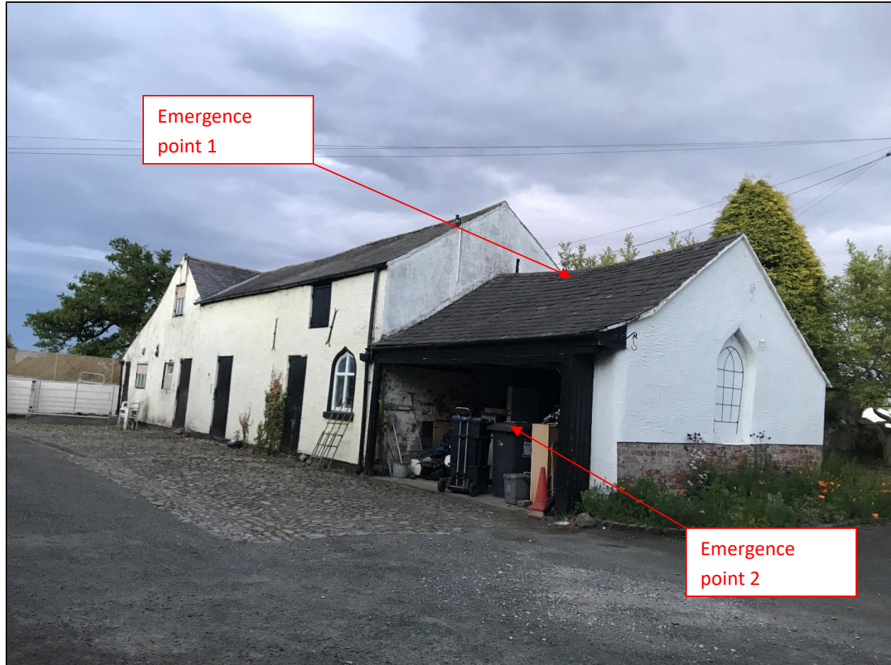
Figure 5.4 - Emergence points 1 and 2 on the south-western elevation of barn, under a roof slate and at the garage door respectively
