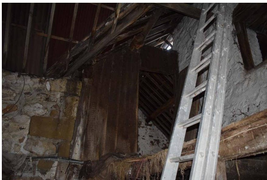
Fig. 15 Loft space above northern room. Inaccessible due to unstable floors. CPAT photo 4950-035
