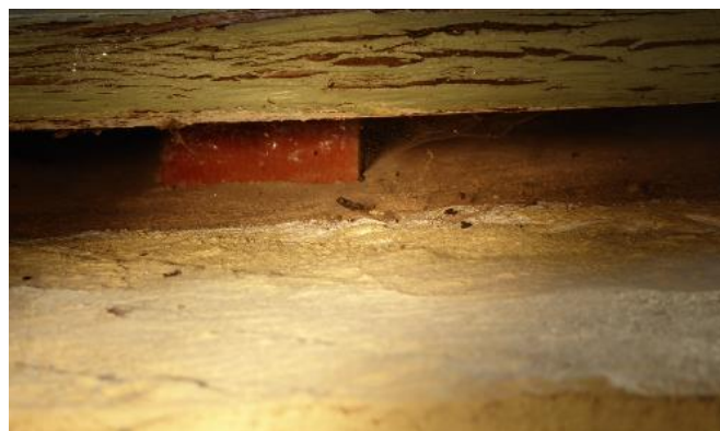
Bat droppings behind the fascia.
