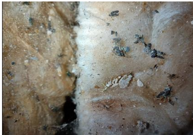
Bat droppings in the loft.
