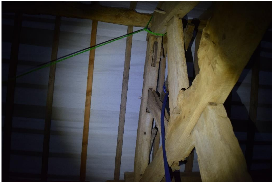
Figure 4.4. Open mortice joint in roof timbers
