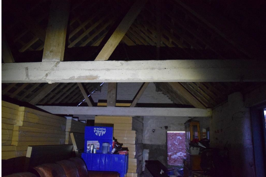
Figure 4.8. Showing gap along western elevation
