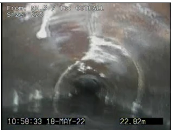
Cracks multiple from 12 to 12 o'clock
