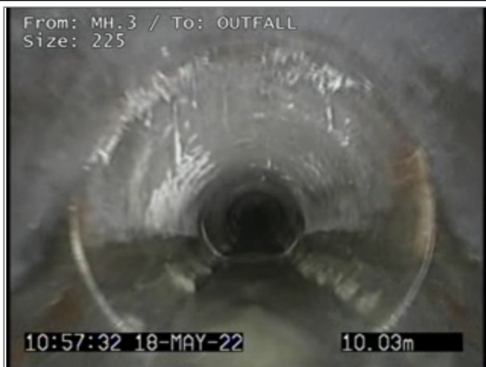
Roots fine at joint
