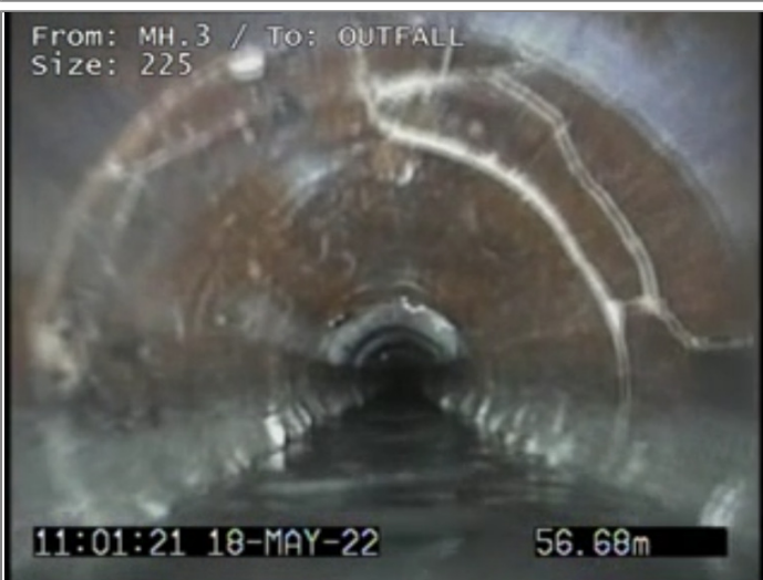
Cracks multiple from 12 to 4 o'clock
