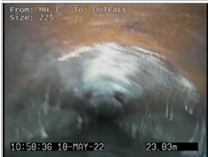
Roots fine at joint
