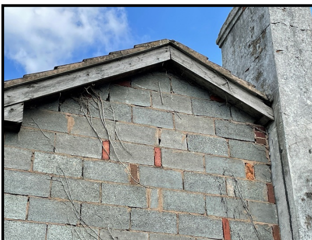
Plate 4 Numerous gaps exist between block-work in B1
