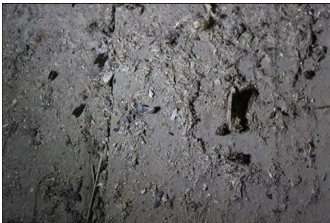
Plate 4 – Evidence of bats ( Pipistrellus pipistrellus ) within the barn mezzanine
