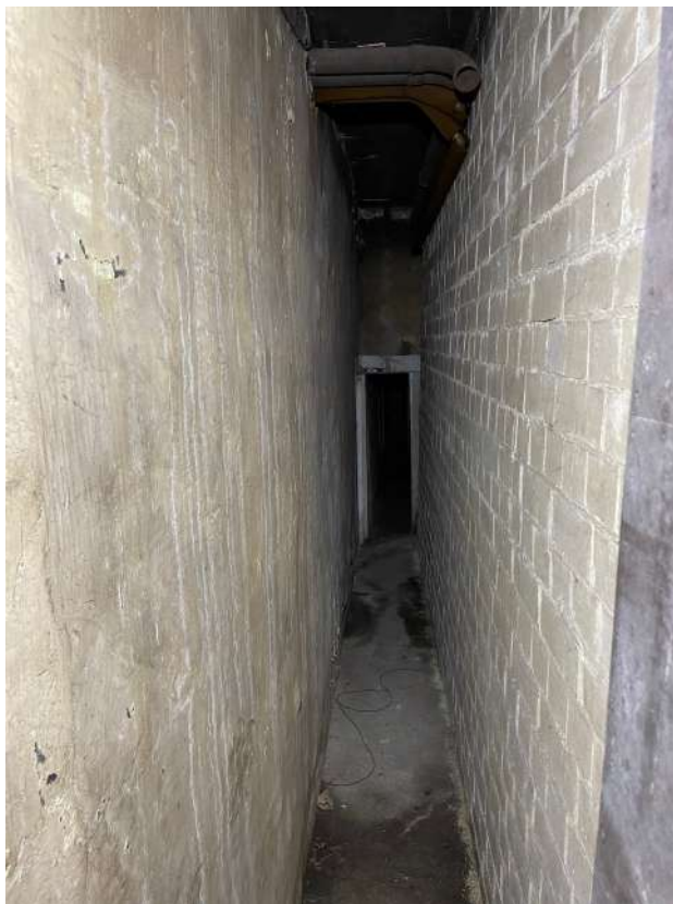
Plate 52 - Void between structure walls and vault
