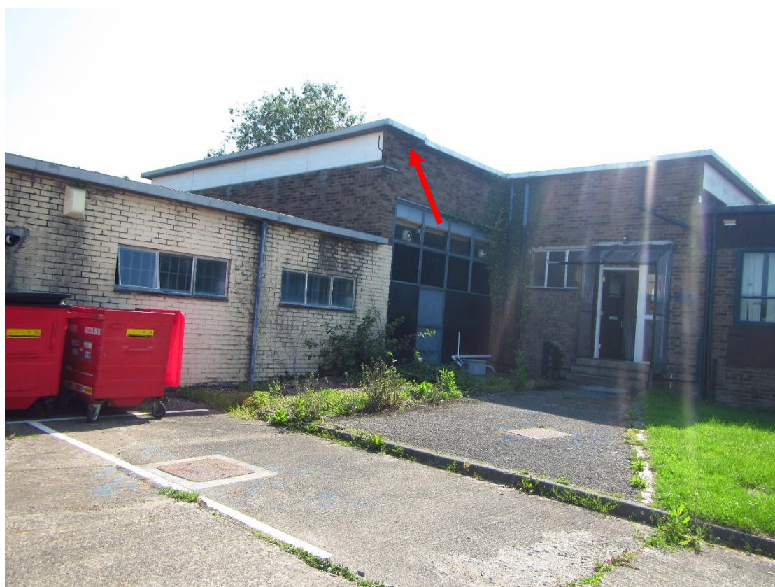
Photograph 4 – Arrow to show location of gap in brickwork.
