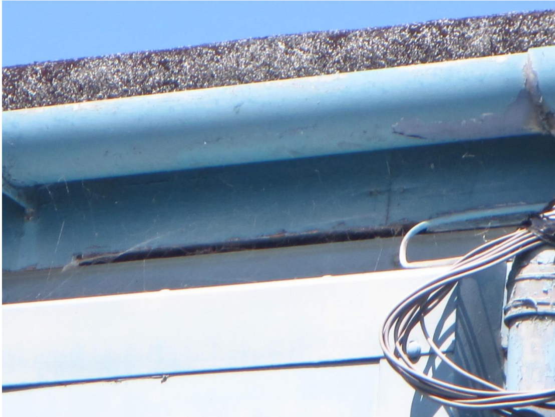
Photograph 15 – Gap in fascia on eastern aspect of Building 4.
