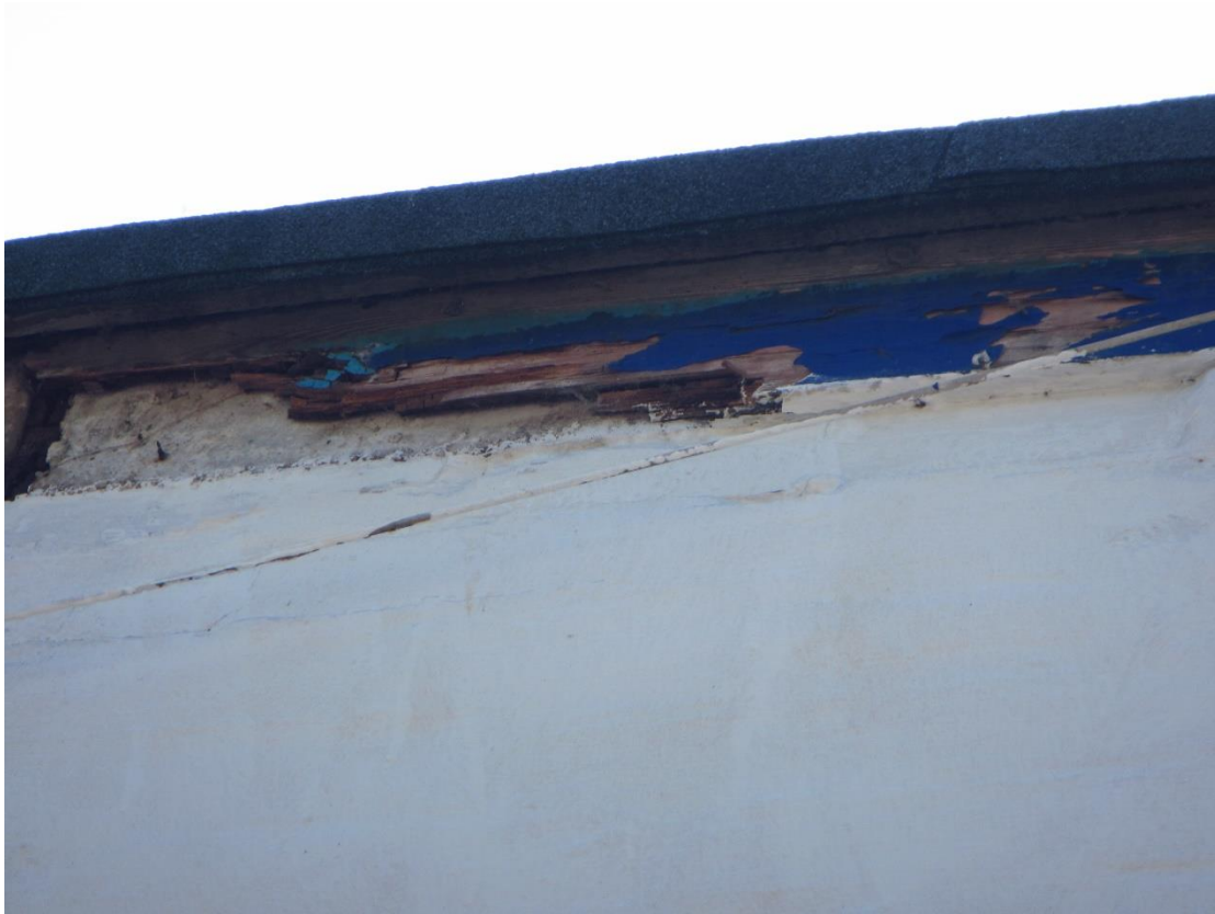
Photograph 9 – Broken fascia board on Building 2, western aspect.
