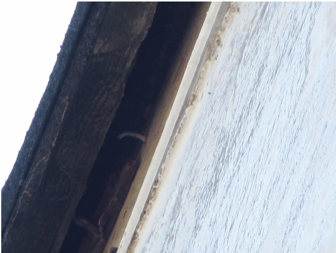
Photograph 10 – Gap in fascia board on Building 2, western aspect.
