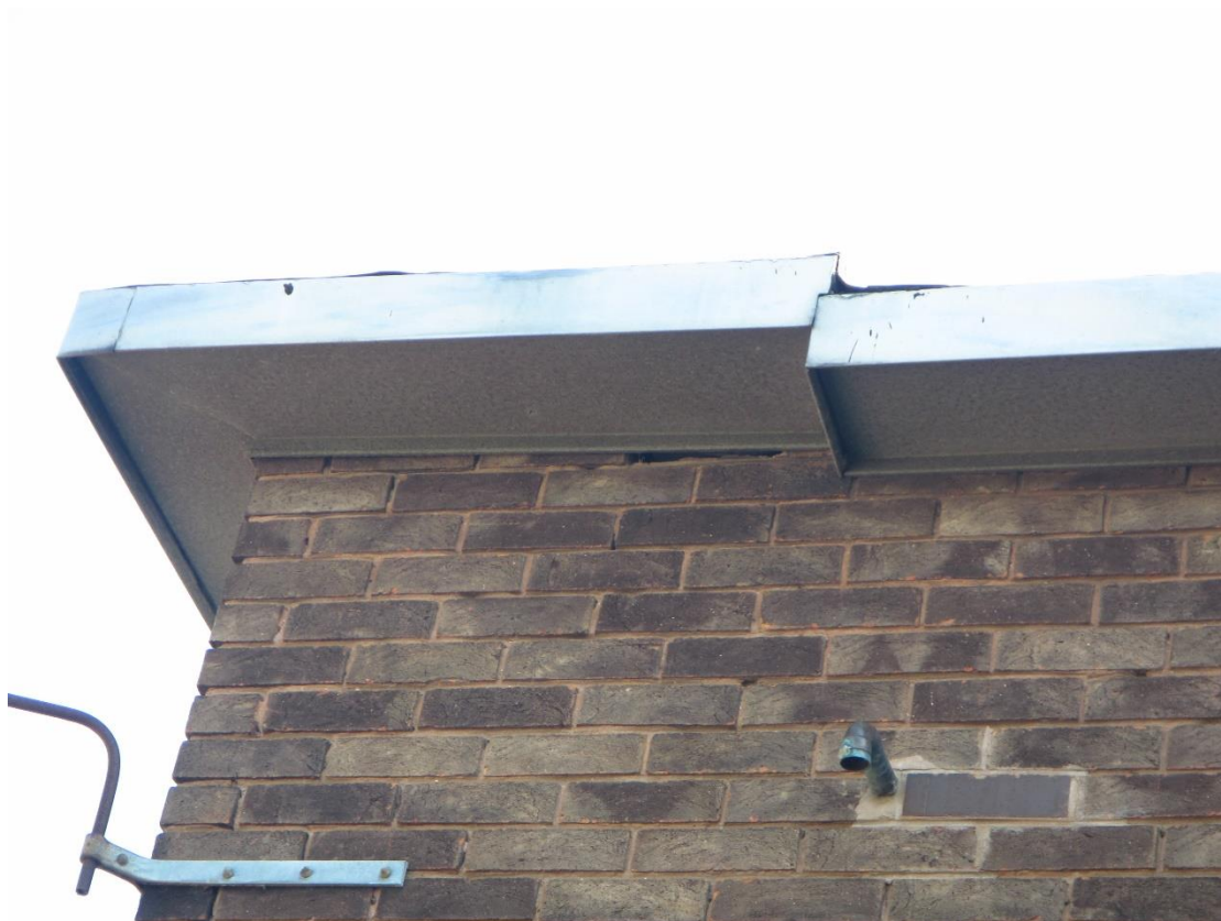
Photograph 3 - Gap in brickwork on southern aspect of Building 1.
