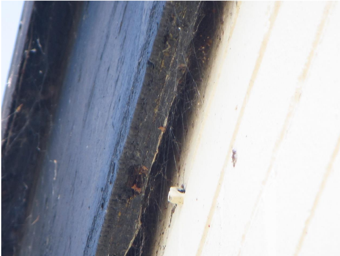
Photograph 17 – Close view of gap in barge board on southern aspect of Building 4.
