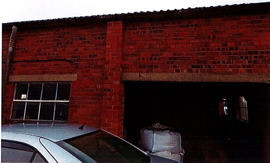
Photograph 1 Showing cracking on side of barn
