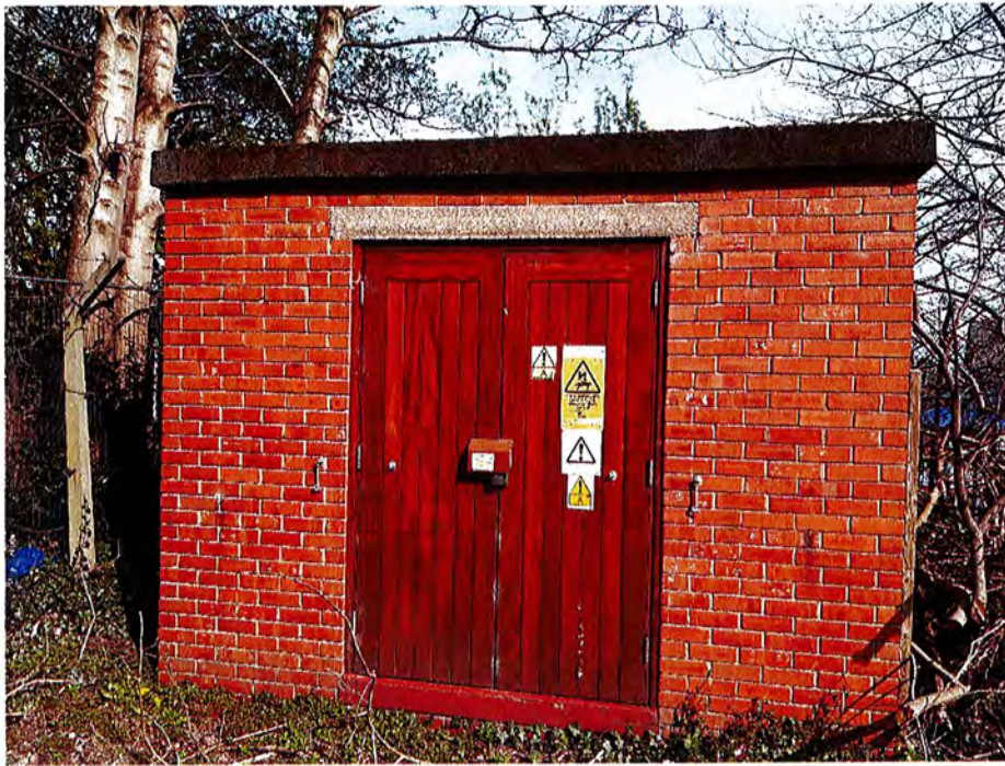
Photograph 5- Facing north showing the substation.
