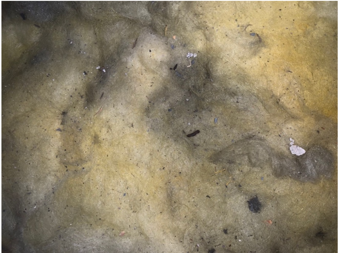
Photograph 4. Bat dropping within roof void
