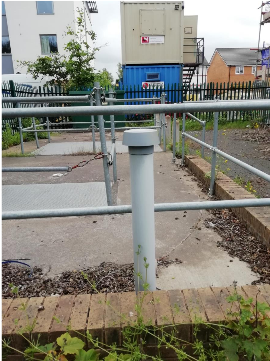
Figure 3-4: Sewage Pumping Station – Picture 4 – showing grey air admittance valve in the foreground
