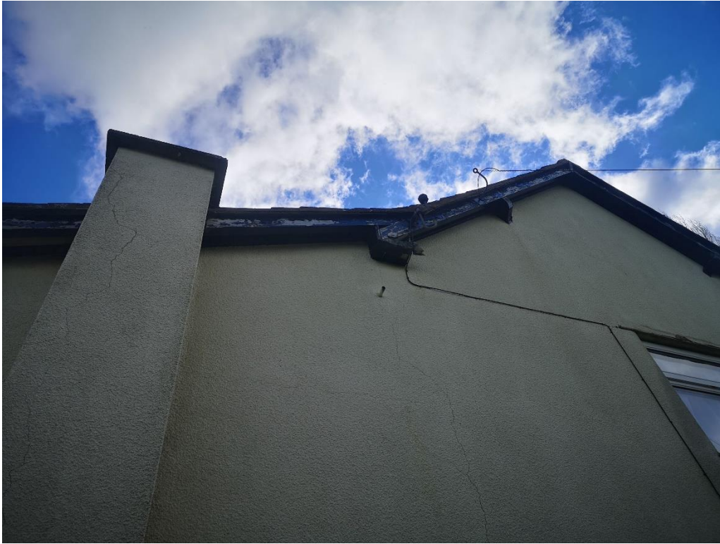
Plate 5 – Large gap in soffit being utilised by house sparrows
