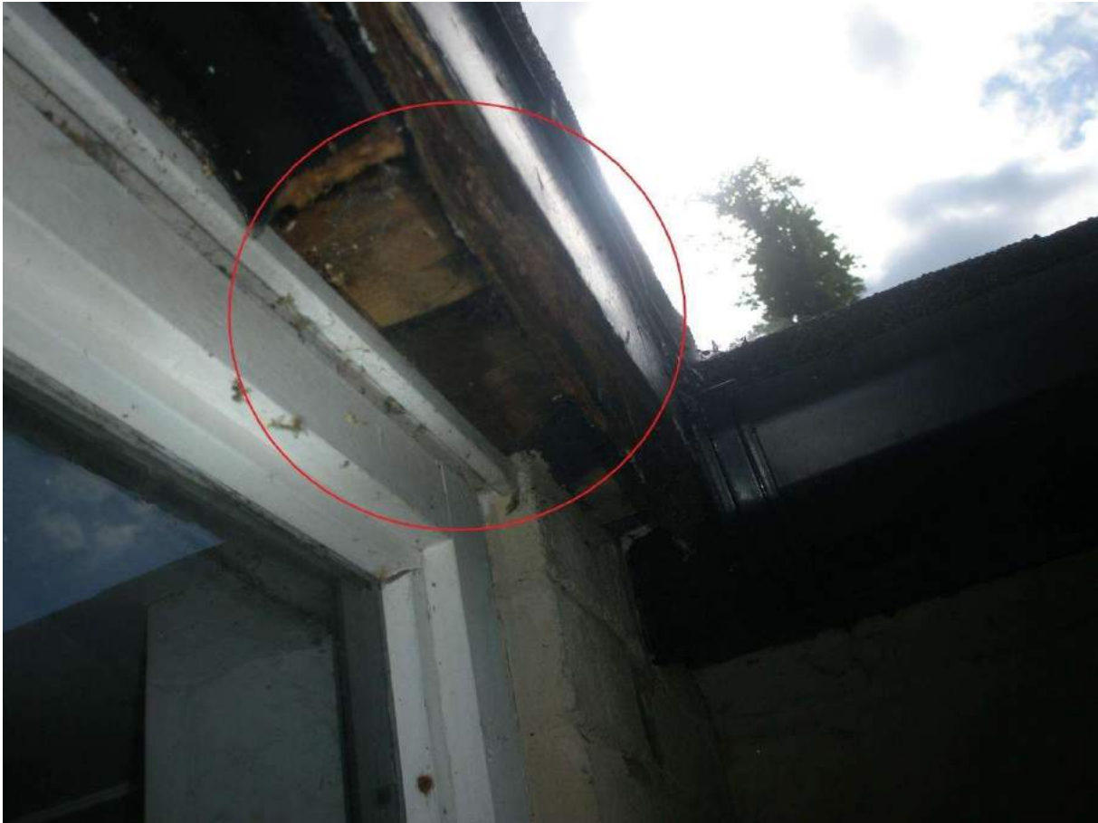
Image 14: Feature 6 as shown in Appendix C, showing gaps in soffit box with limited cobwebs present.
