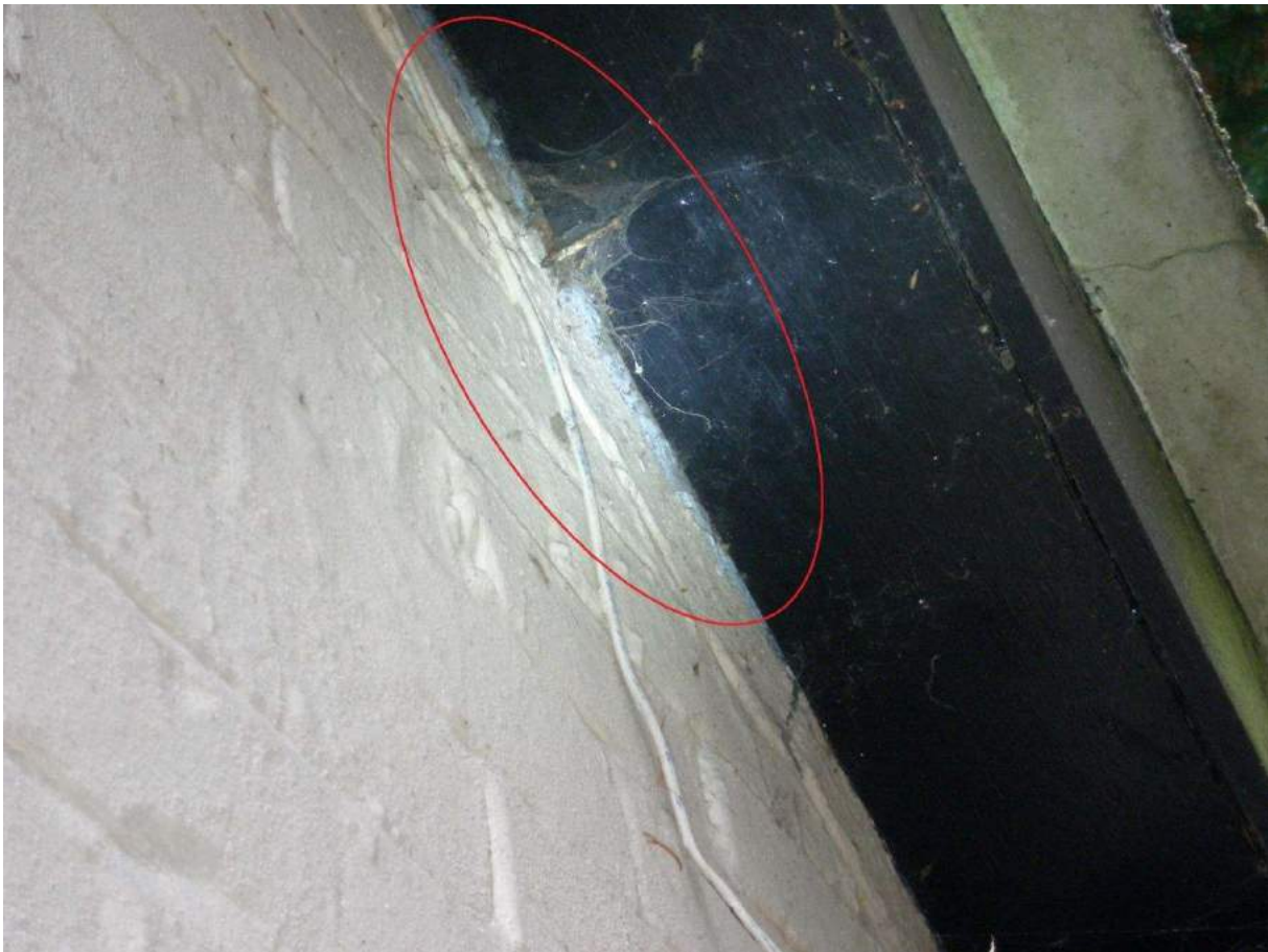
Image 9: Feature 1 as shown in Appendix C, showing gaps under gable soffit box with cobwebs present.
