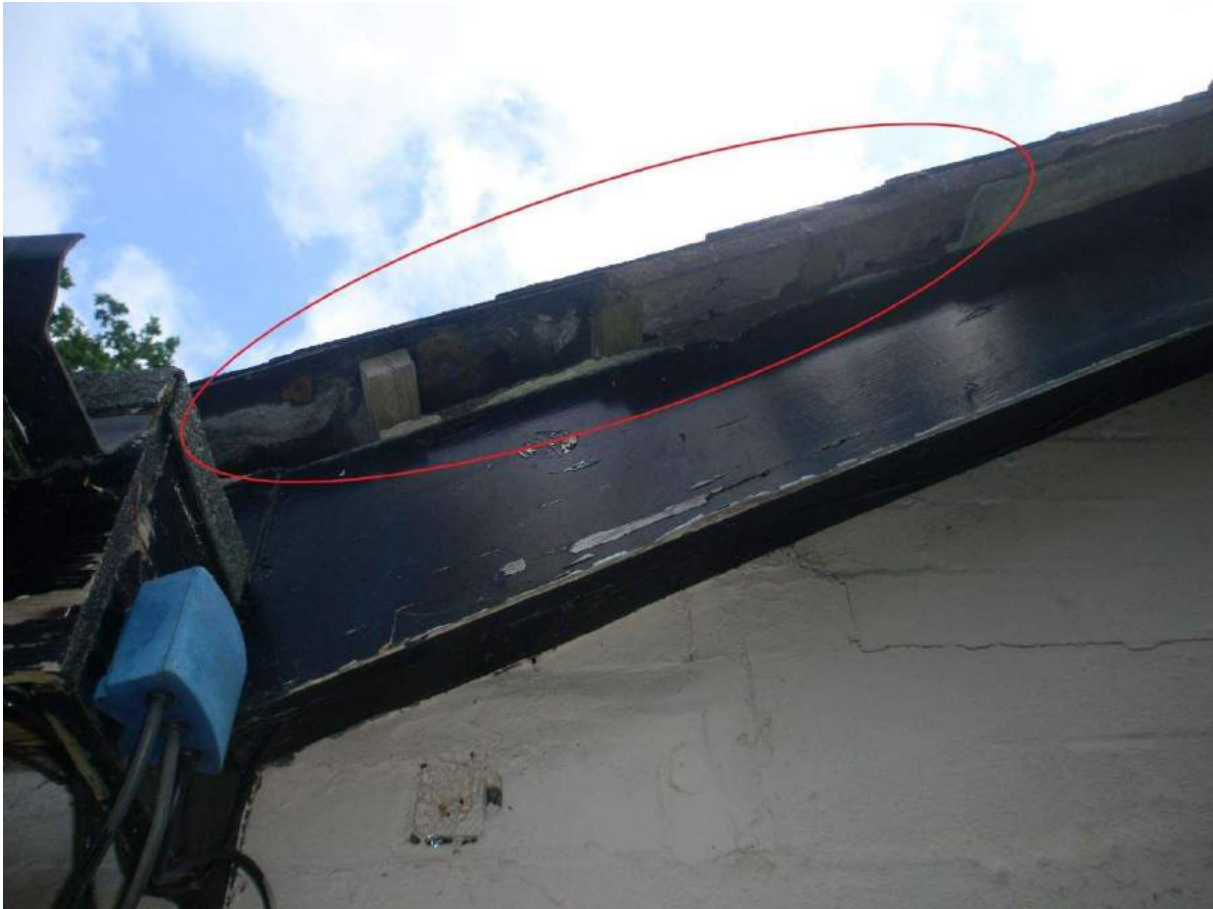
Image 17: Feature 9 as shown in Appendix C, showing gap under soffit box at gable end and ridge joint with limited cobwebs present. Tile pointing also missing with gaps present.
