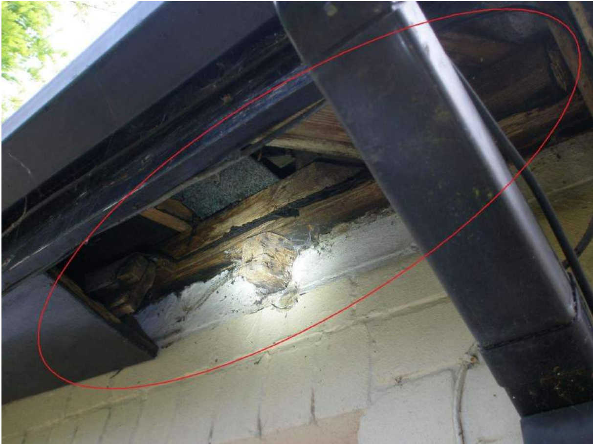
Image 16: Feature 8 as shown in Appendix C, showing panel out on soffit box.
