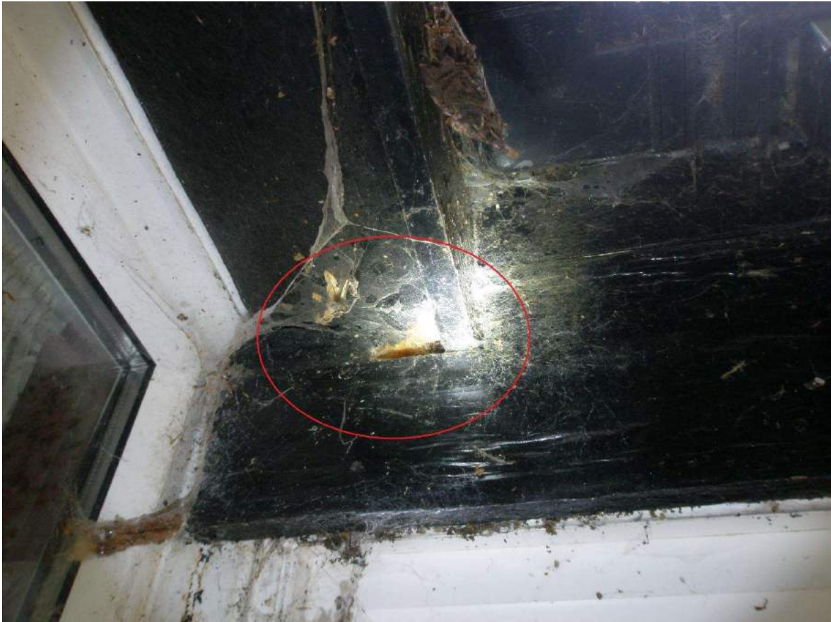
Image 11: Feature 3 as shown in Appendix C, showing gap where soffit box meets structure extension with cobwebs present.
