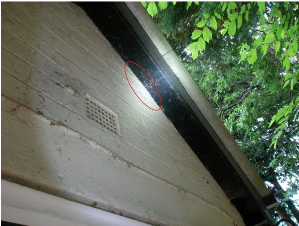
Image 10: Feature 2 as shown in Appendix C, showing gaps under gable soffit with cobwebs present.
