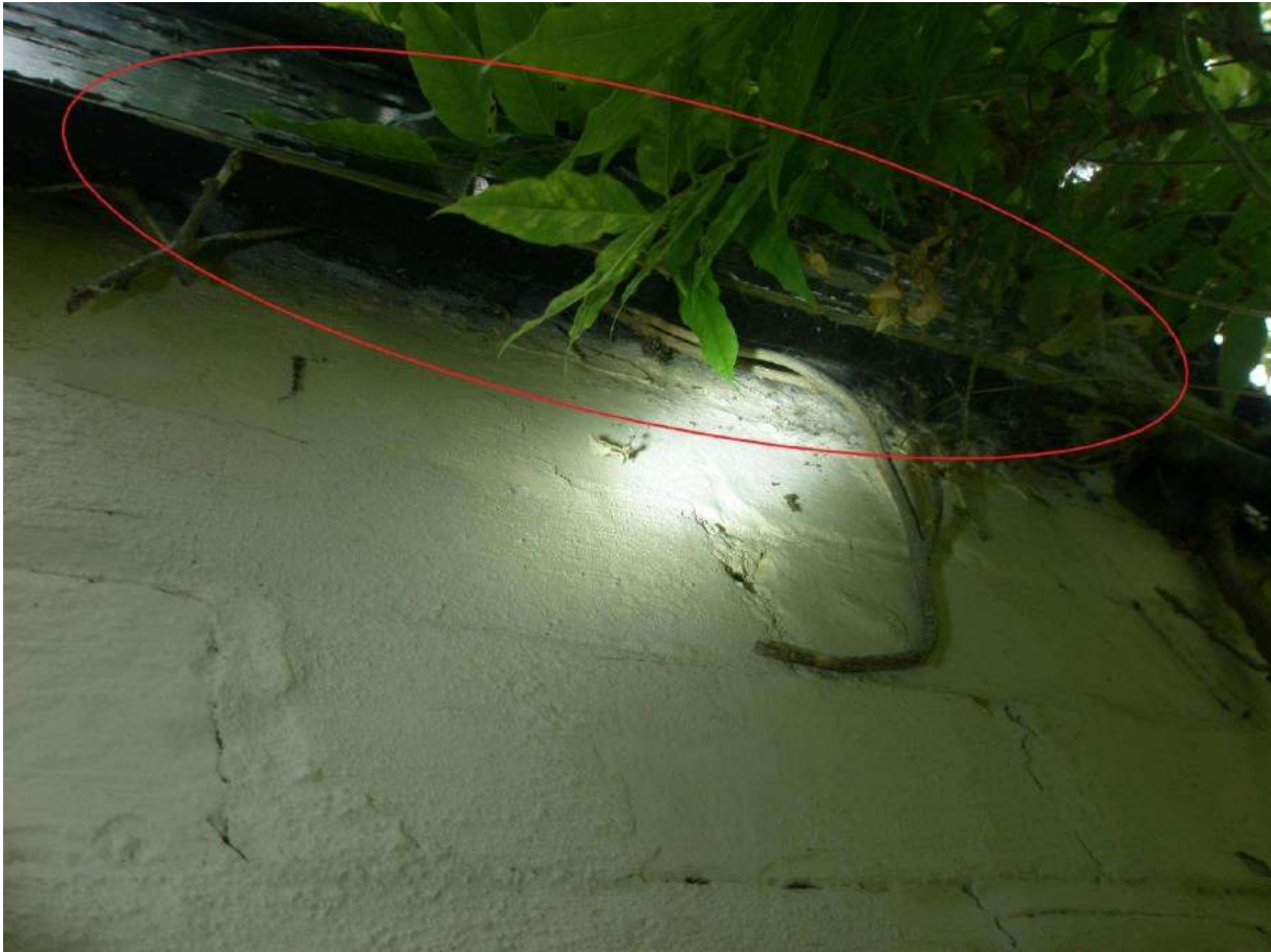
Image 15: Feature 7 as shown in Appendix C, showing gaps under bargeboard with limited cobwebs present.
