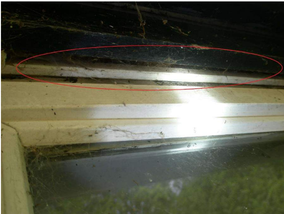
Image 13: Feature 5 as shown in Appendix C, showing gaps under bargeboard with cobwebs present.
