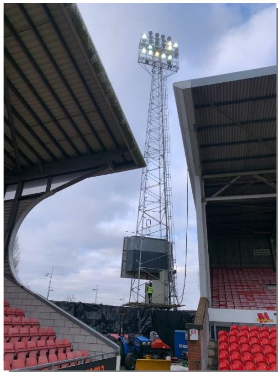
Figure 2. Photo for the existing floodlights
