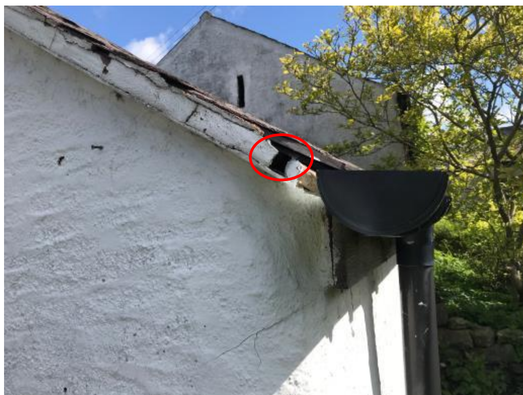
Plate 4 – Viewed from the south with a gap in the mortar at the roof verge indicated
