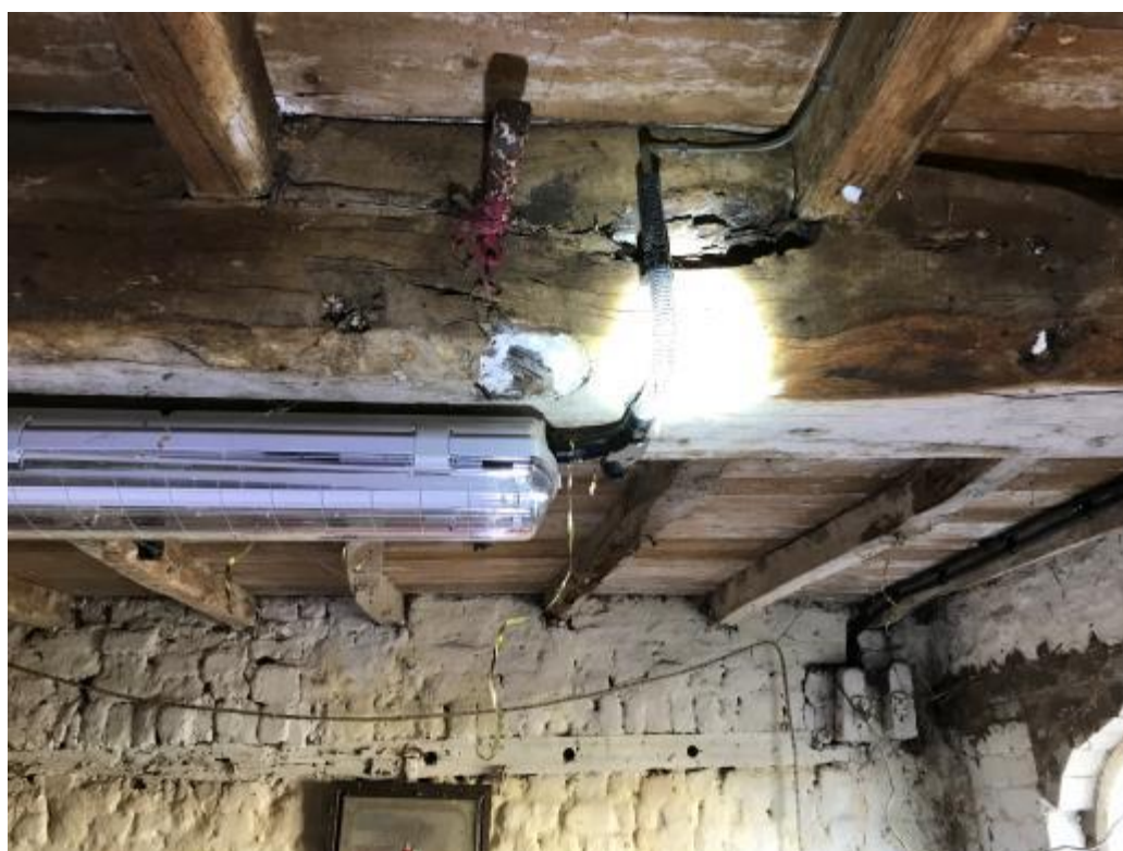
Plate 14 – Crevices in internal timbers
