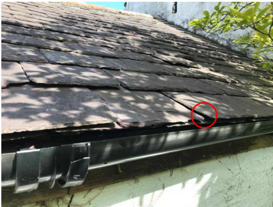
Plate 5 – Gap beneath lifted slates
