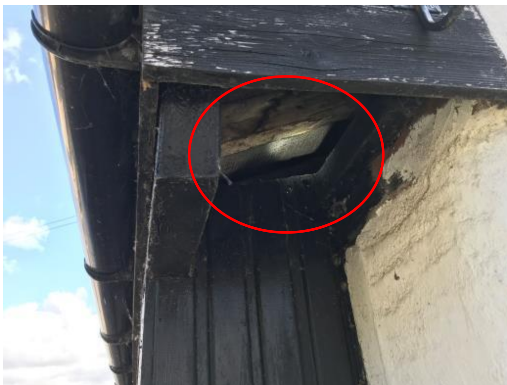
Plate 6 – Gap in the wooden soffit box
