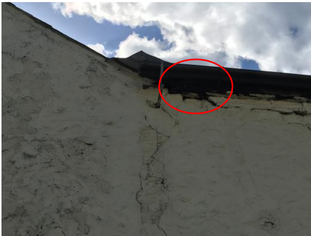
Plate 7 – Crack at roof-verge
