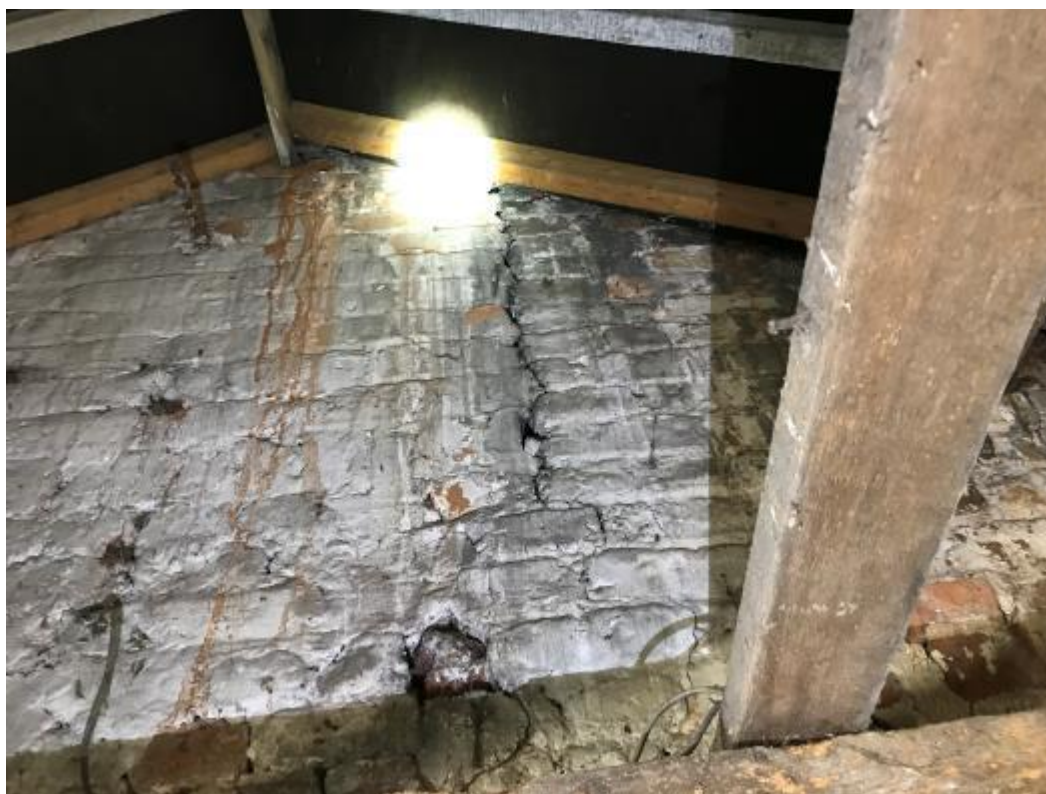
Plate 15 – Internal crevice in brickwork
